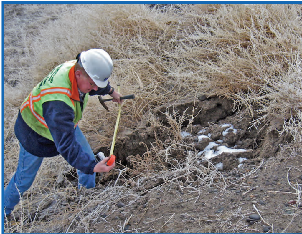
Landside, left canal bank, about 240 feet downstream from the Truckee Canal breach. Collapse feature associated with downhill sediment transport. Three muskrat burrows on the canal side of the embankment near high water line. See the Truckee Canal breach information on the following page.
