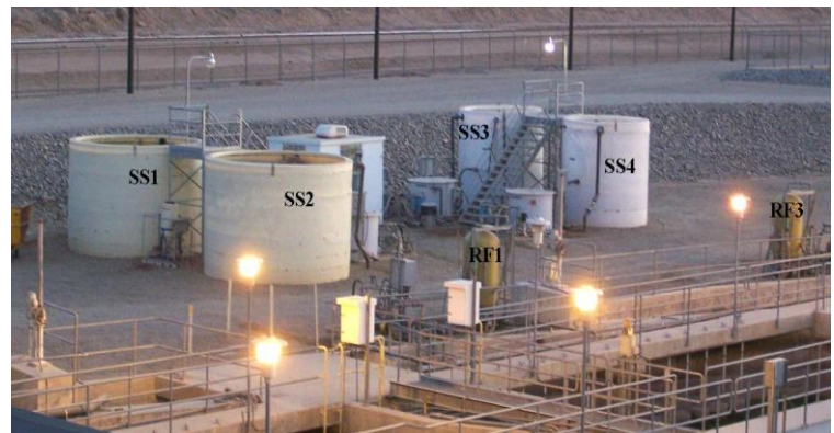
Slow sand filter pilot testing at Reclamation’s WQIC
