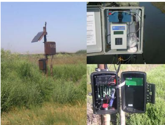
Real-time telemetered flow and salinity monitoring stations.
