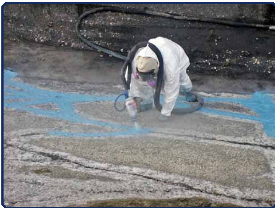
Typical equipment used to apply Aqualastic® in cracks at Roza Canal, Washington, during annual maintenance. (Note that this was not part of the test research project.)
