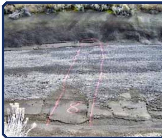
Before: Deteriorating lining from dozer tracks and previous patchwork at the toe of the slopes is typical in this area of the North Unit Main Canal, Oregon.
