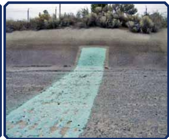
After: The test section after one irrigation season and one winter season. Adhesion to the concrete substrate is excellent and there is no cavitation damage on the coated section.
