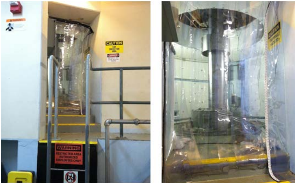
Figure 5. Acoustical barrier between turbine pit and penstock area at Green Springs Powerplant.
