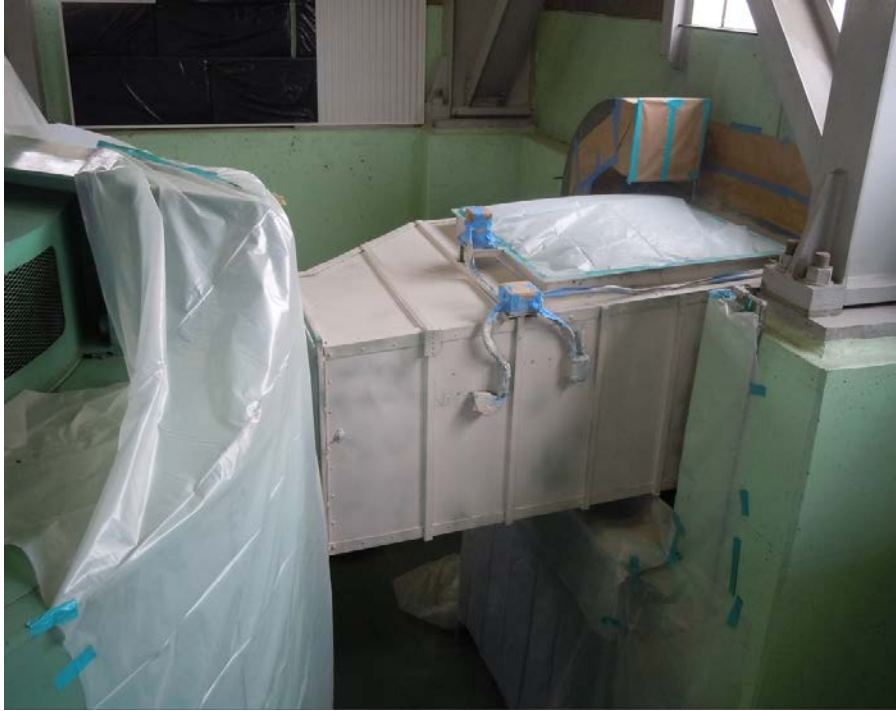
Figure 7. Spray-on damping material on cooling ducts at Roza Powerplant.
