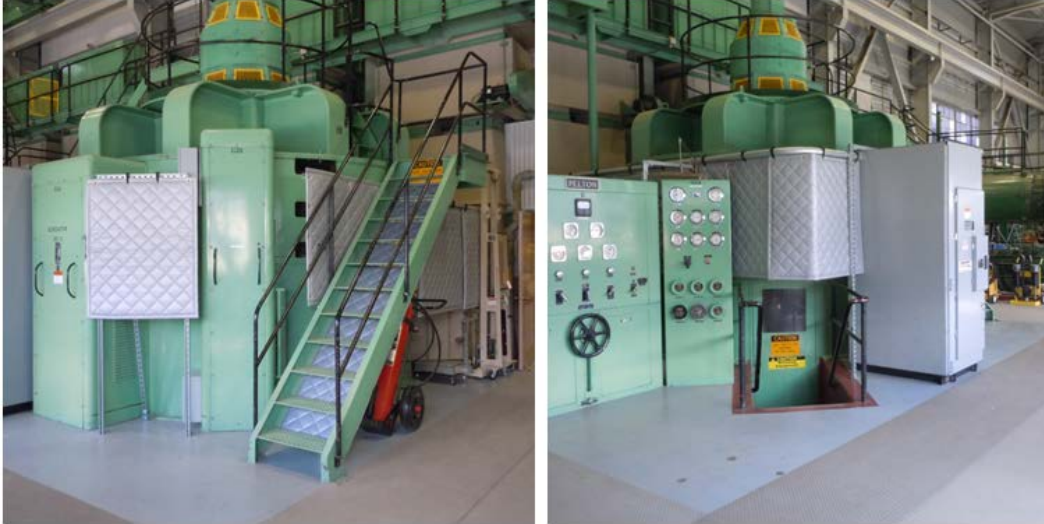
Figure 6. High transmission loss acoustic barrier in front of the generator cooling slots.
