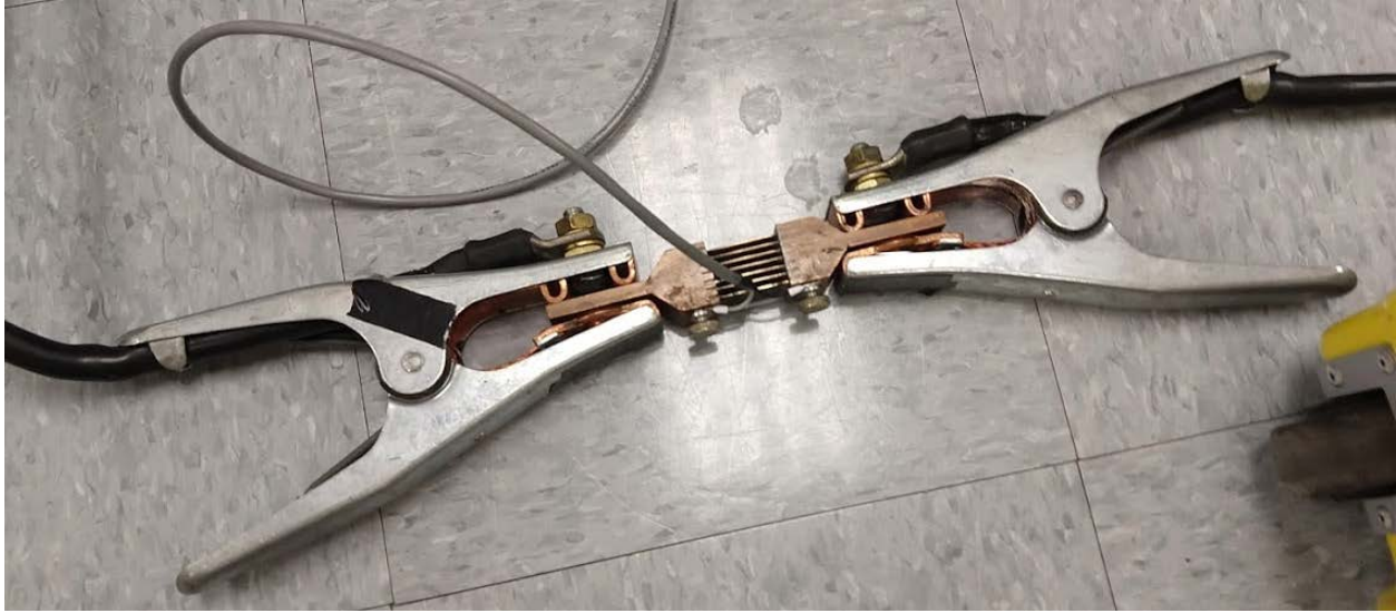
Figure 2.—500 A to 50 mV shunt in primary circuit
