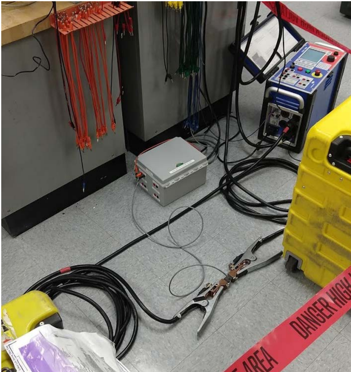
Figure 1.—CPC 100, current path (cables), and shunt Note: OCT just off picture to top right, intentionally left out of photo
