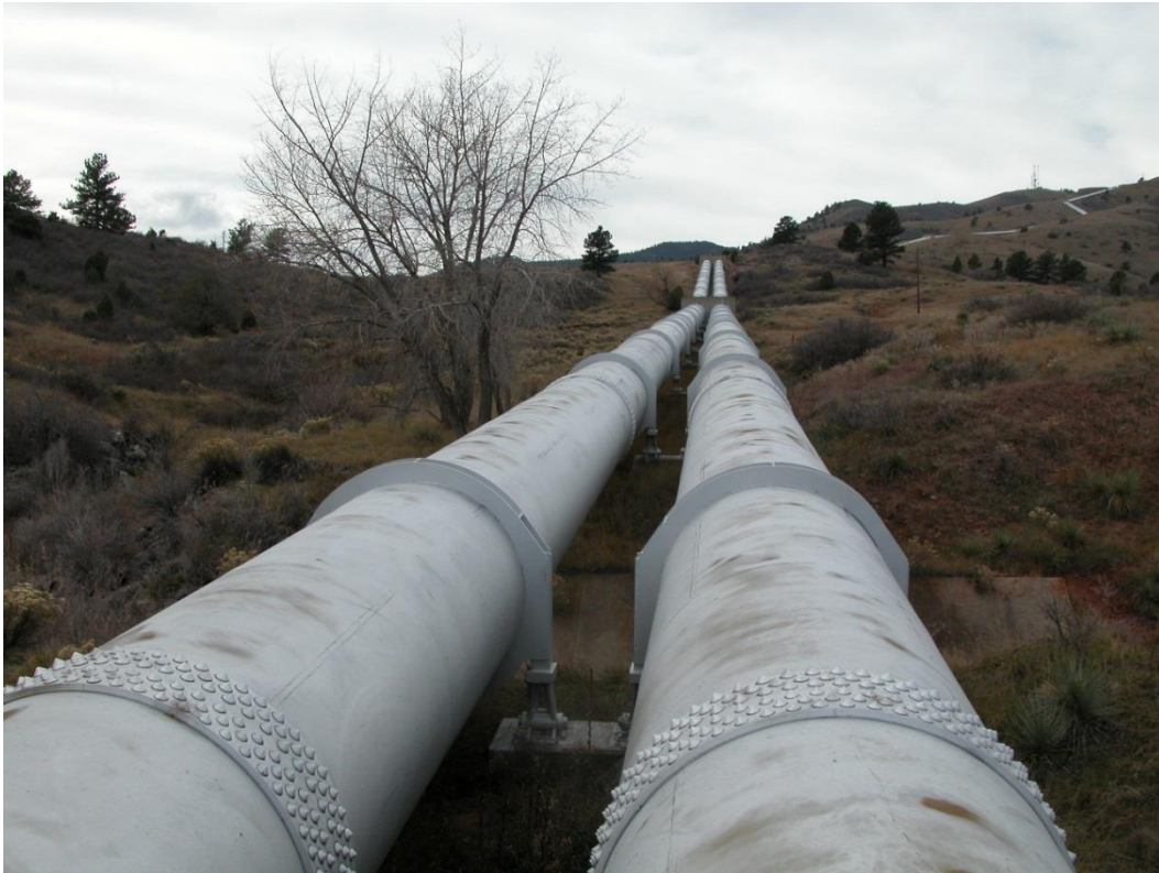
Figure 2: Lead-coated penstock exteriors at Flatiron Powerplant in 2007. The exteriors were recoated with a zinc-rich primer and polyurethane topcoat in 2010.
