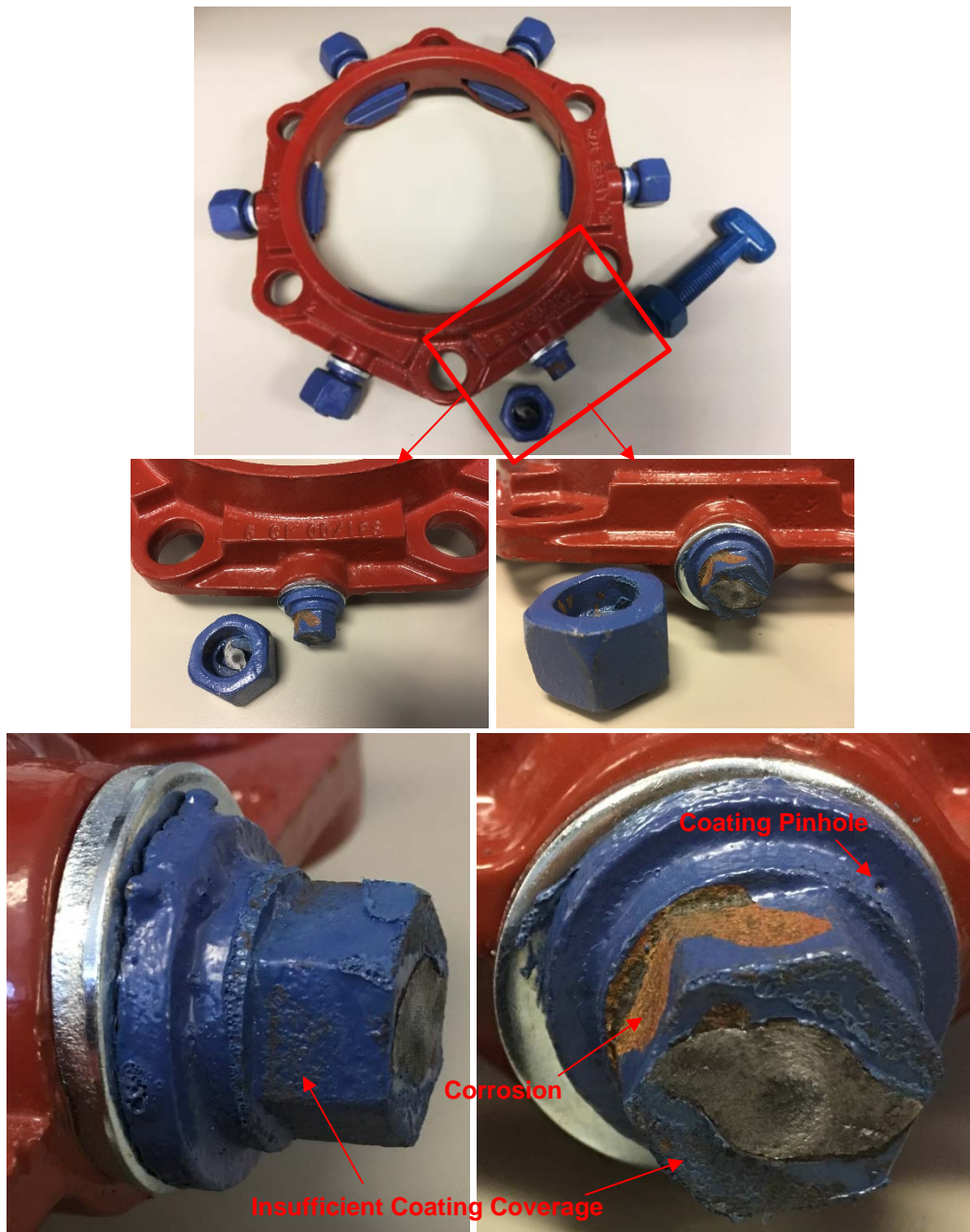
Figure 20.—Sheared-off nut and remaining hex nut; corrosion seen inside nut and on the hex nut. In addition, pinholes in the coating and insufficient coating coverage observed at various areas on the hex nut.
