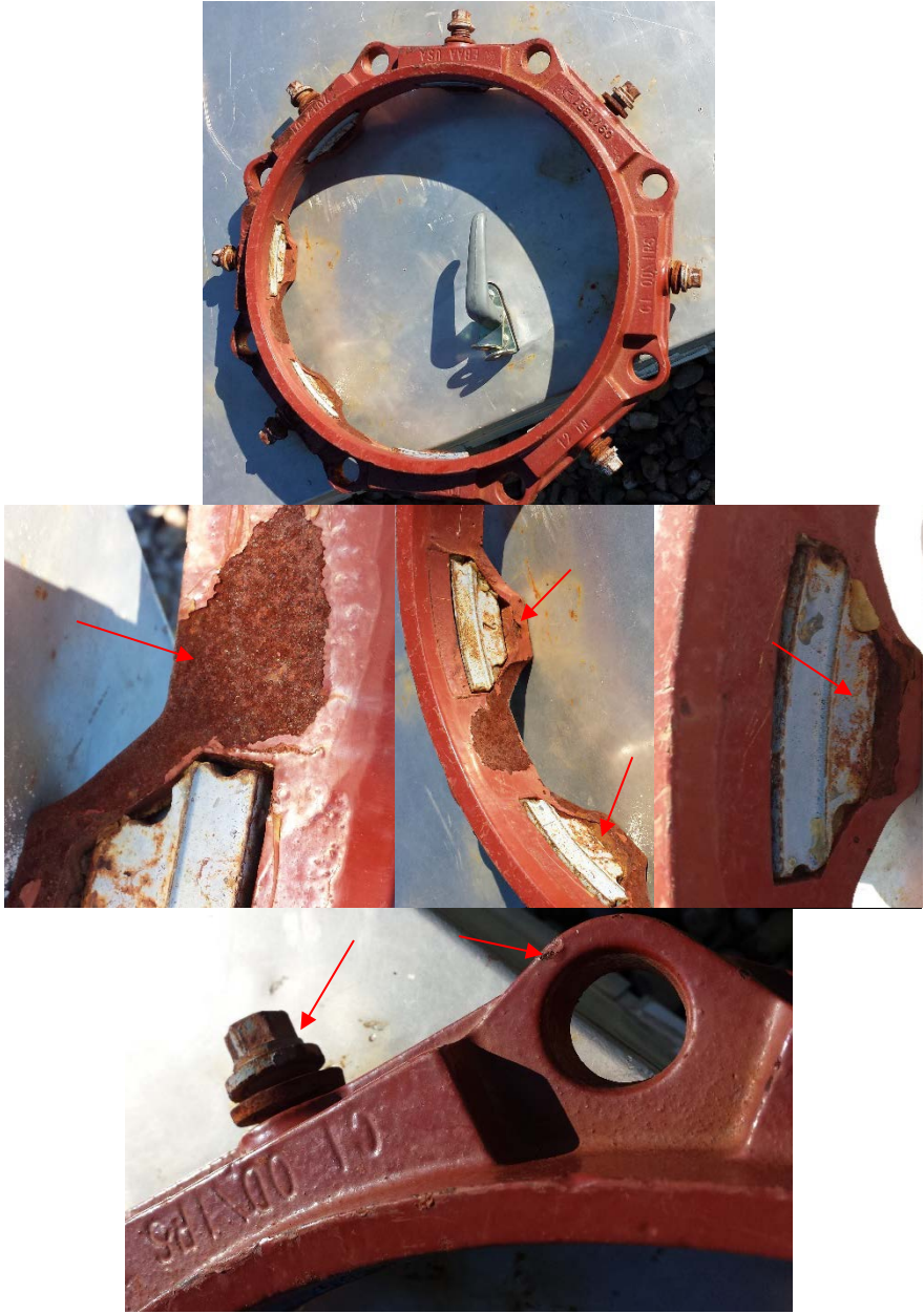
Figure 21.—Failed mechanical joint restraint used for Pine Ridge Oglala Sioux Tribe Reservation Pipe (7 to 8 years in service). Coating damage and corrosion seen at different locations.
