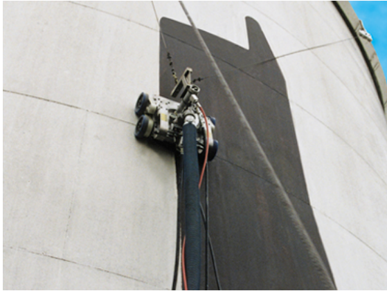
Figure 3. Flow corp vacuum crawler
