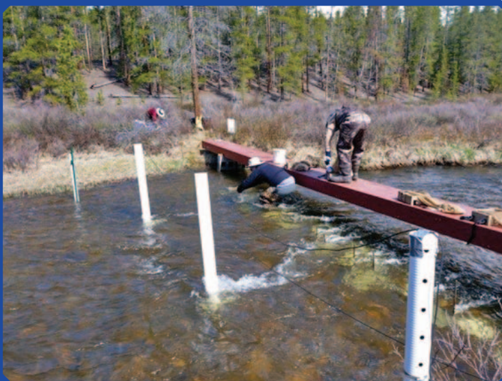
Installing Bunte bed load traps immediately downstream of two hydrophones on Halfmoon Creek, Colorado. The hydrophones are installed near the bed using posts and hydrodynamic fairings.
