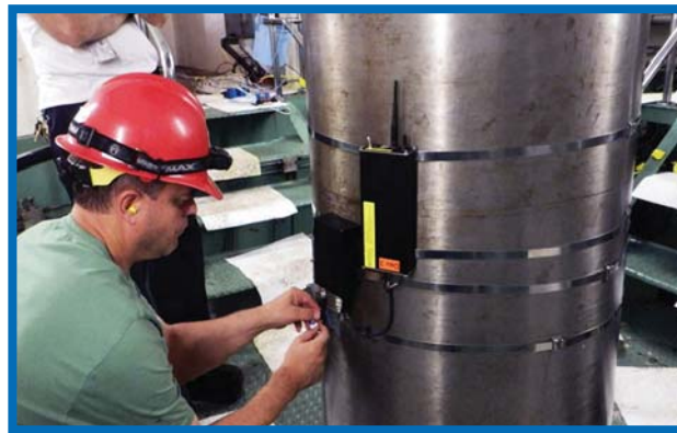
Jim DeHaan of Reclamation’s TSC installing a cavitation monitor at the J.F. Carr Powerplant.
