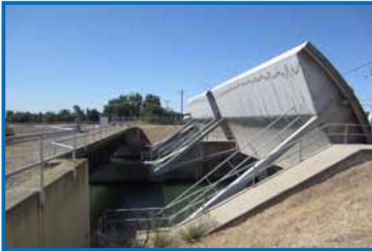
Delta Cross Channel gates in the open position, California.
