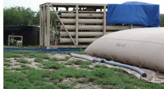
The EUWP stores purified drinking water.
