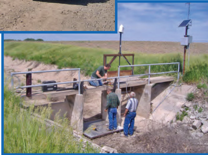
In the bottom right photo, Bostwick personnel are installing an overshoot gate that was fabricated in the district's shop as part of the demonstration.
