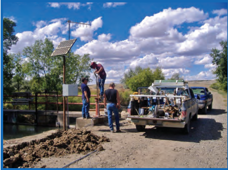
In the left photo, Buford-Trenton ditch-riders are installing a gate motor at the end of system spill site.
