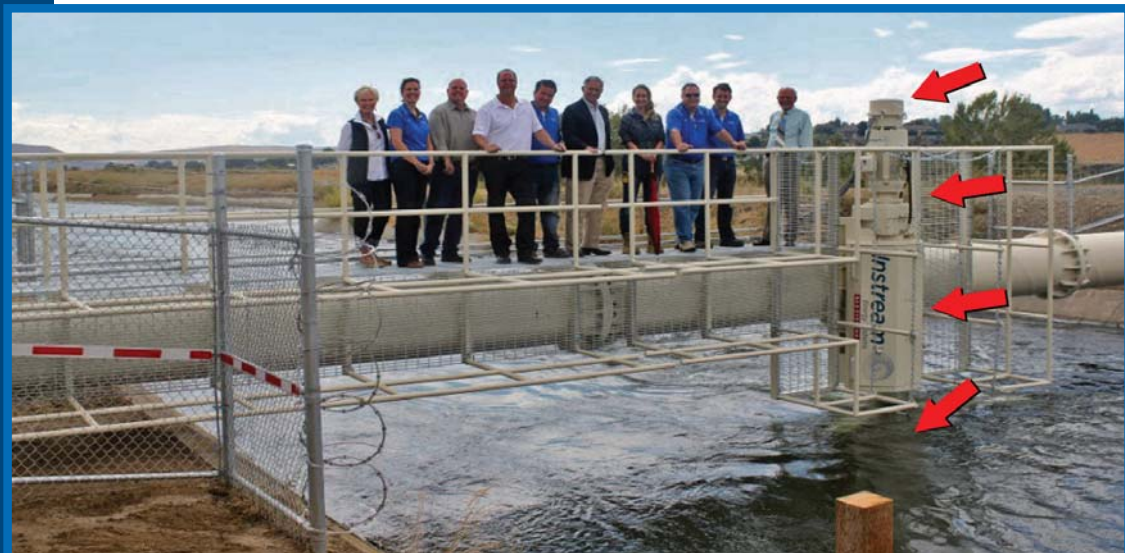
The HK device is attached to a spanning structure that is secured to both sides of the Roza Canal on concrete foundations. The spans prevent contact with the existing canal structure to preserve the physical integrity of the canal lining, as well as ongoing operations. Visitors to the site (left to right): Jane Shaw, Canadian Consulate Seattle; Shannon Halliday, IES; Sid Ottem, Reclamation; Brett Hawse, IES; Ken Miller, IES; Phil Georgariou, BAE Systems; Ali Grovue, IES; Jim Hawse, IES; Shane Grovue, IES; and Congressman Doc Hastings.
