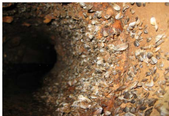
Quagga mussel infested power plant cooling water pipe.
