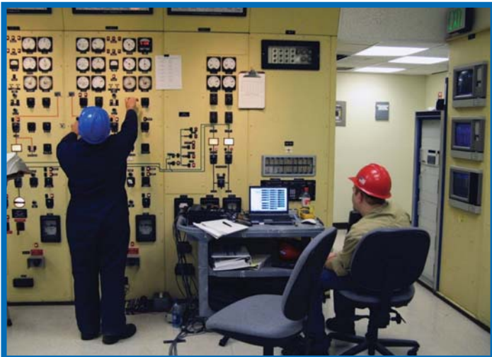
The control room at Flatiron Powerplant, Colorado-Big Thompson Project, Colorado.
