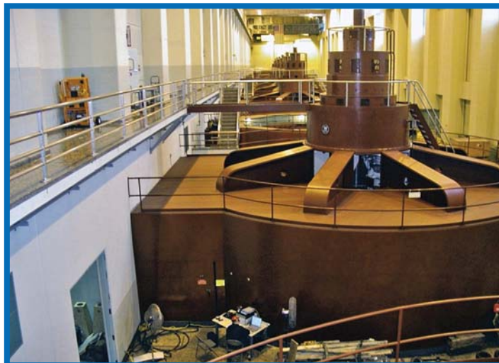
Right Powerhouse, Grand Coulee Dam, Columbia Basin Project, Washington.
