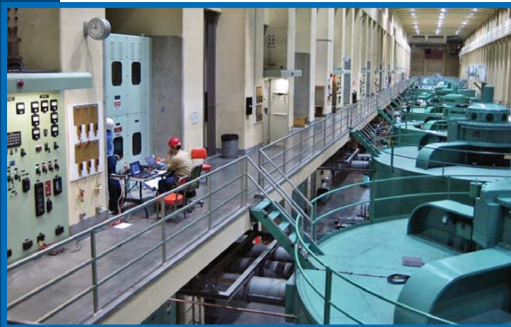
John W. Keys III Pump-Generating Plant, Grand Coulee Dam, Columbia Basin Project, Washington.
