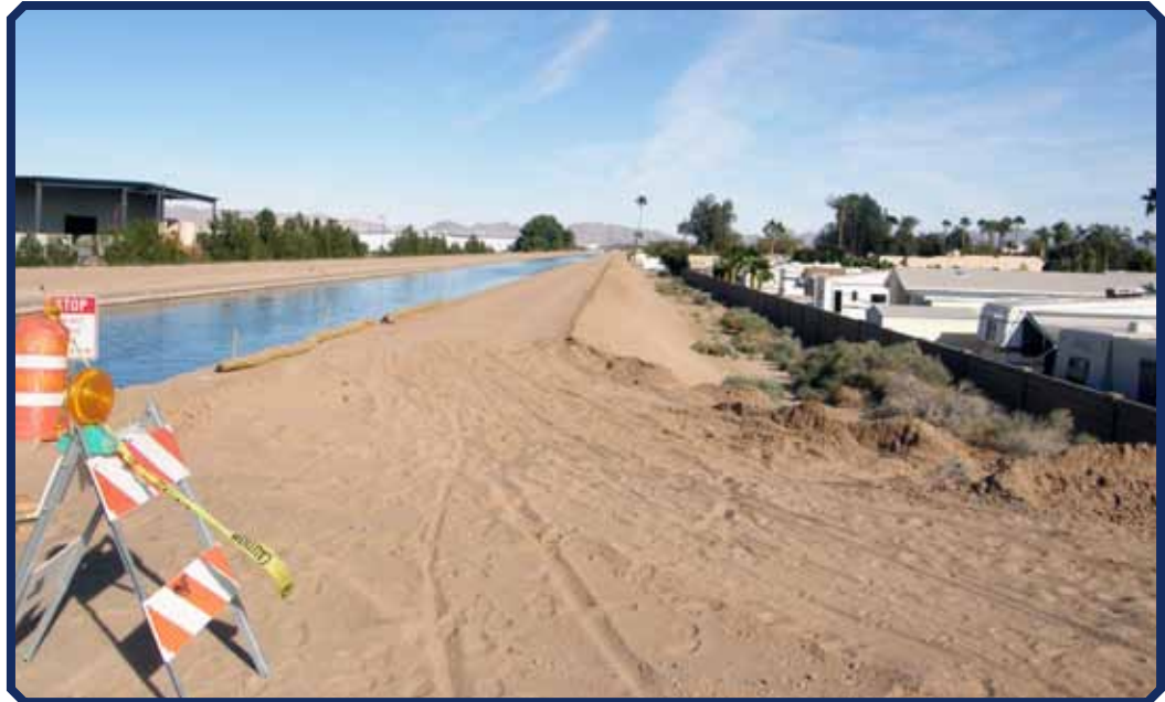
Example of a canal of concern, highlighting that some of Reclamation's canals are above urbanized populations.
