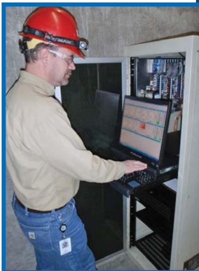
Jim DeHaan of Reclamation's TSC installing and configuring the machine condition monitoring system at Grand Coulee Powerplant, Washington.
