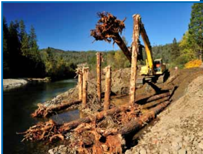
Large wood structure under construction at the Sawmill Rehabilitation Project (2009) on the Trinity River, near Lewiston, California.
