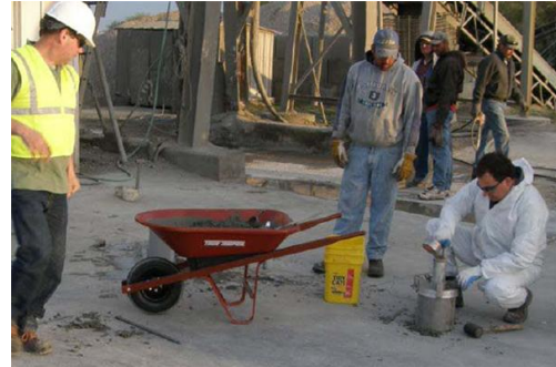
Measuring fresh properties of the concrete after adding the Premier Magnesia additive.
