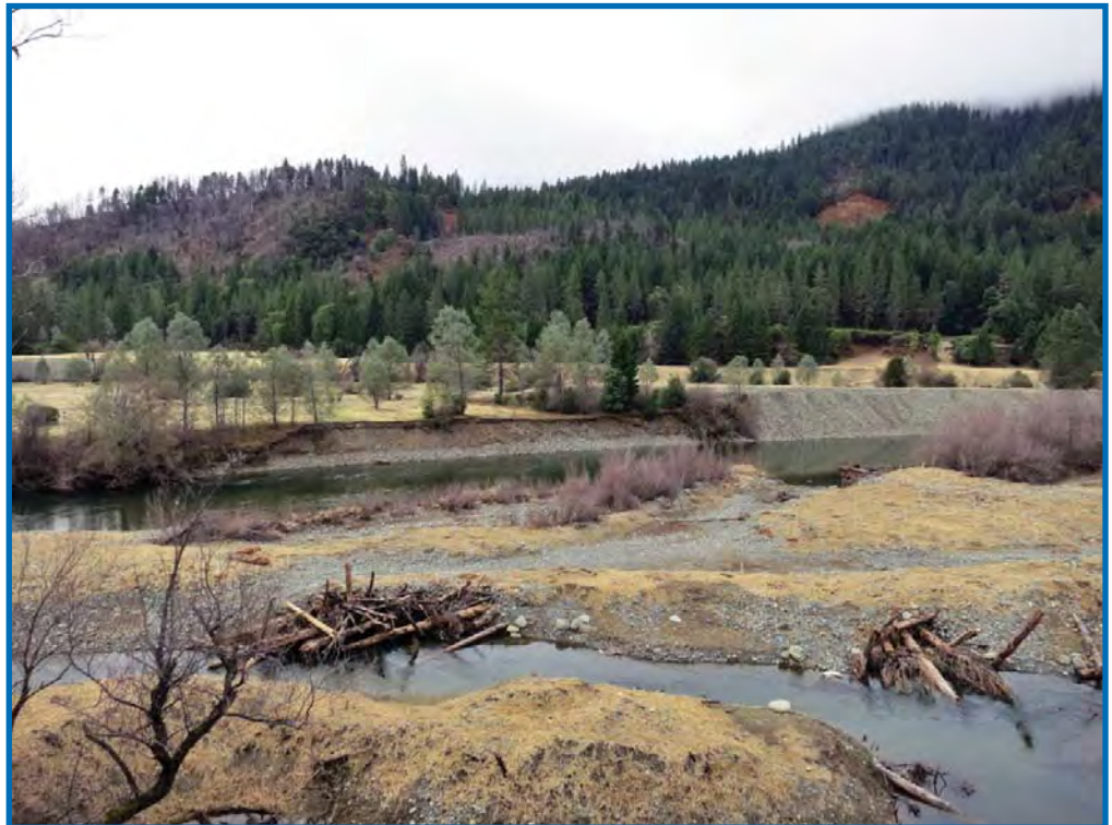
Channel restoration project on the Trinity River near Upper Junction City, California. A constructed side channel for the purpose of increasing salmon rearing habitat is in the foreground and an eroding bank is behind it.
