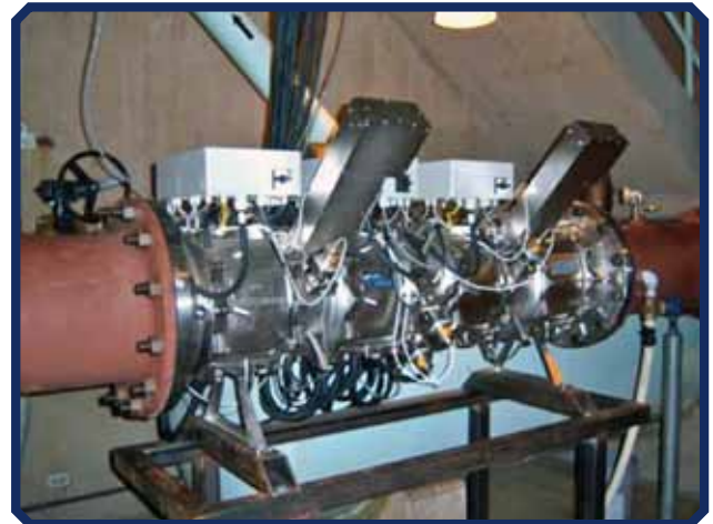
UV unit installed at Davis Dam (Arizona/Nevada) for mussel treatment.
