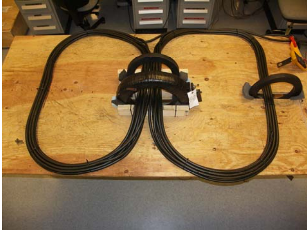
Figure 2 – Grand Coulee Powerplant - CT Calibration (Fourteen loops of cable pass through both the larger plant CT and smaller standard CT located in the middle of the table.)
