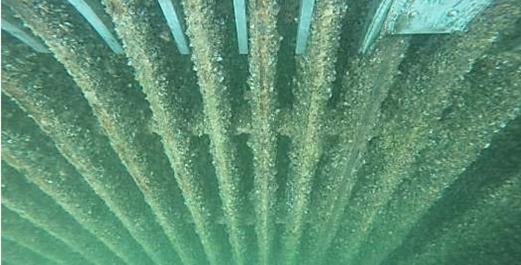
Figure 14.—Existing coal tar enamel coated trashrack.
