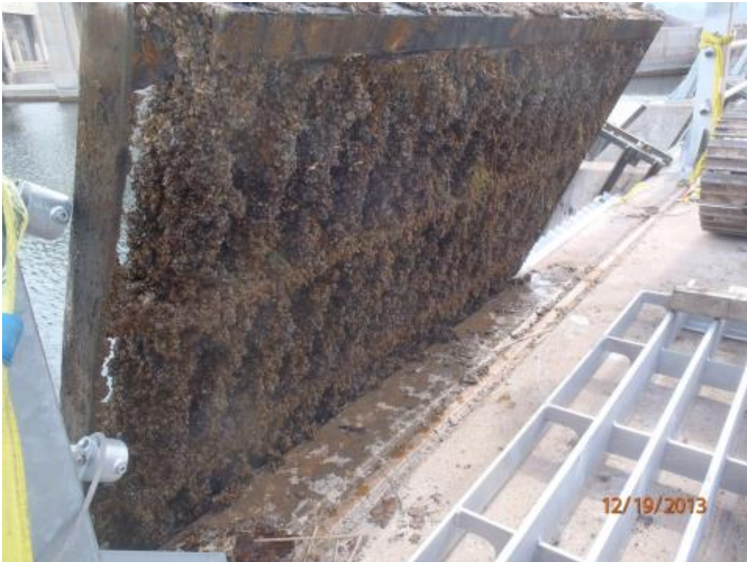
Figure 1.—Existing trashrack heavily fouled with quagga mussels.
