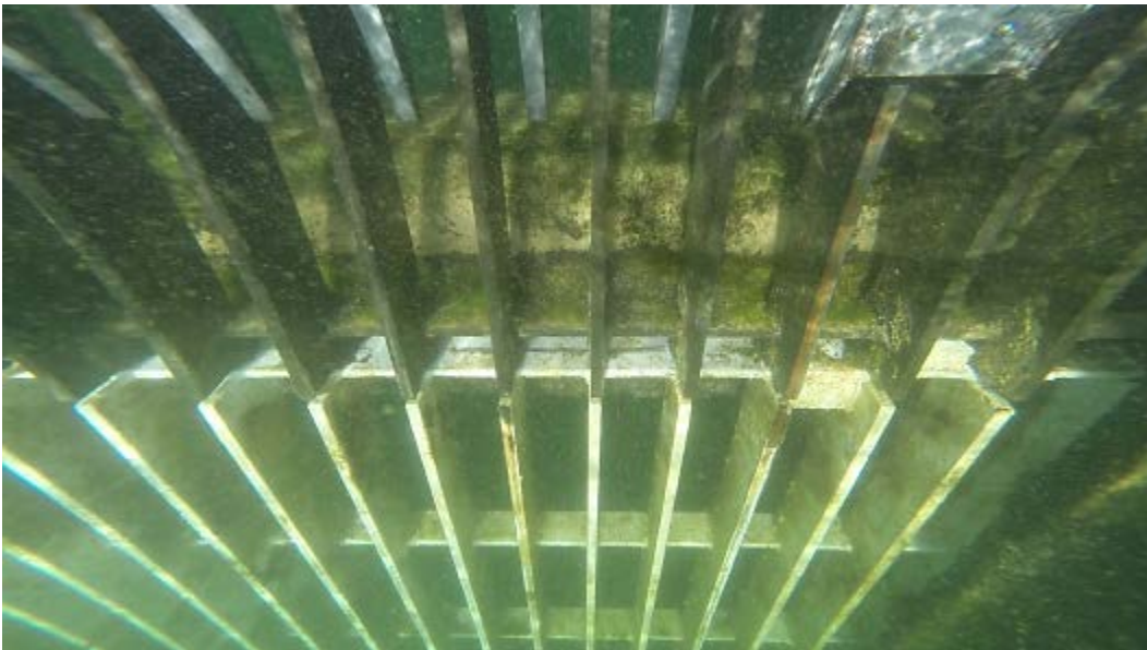
Figure 13.—New galvanized trashrack panel shows corrosion on leading edge where trash rake guide scrapes the surface (third bar from right).
