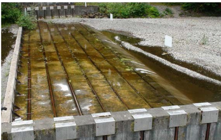
Figure 2. Example of an electric barrier with bottom flush-mounted electrodes at Quinault Fish Hatchery, Washington.
