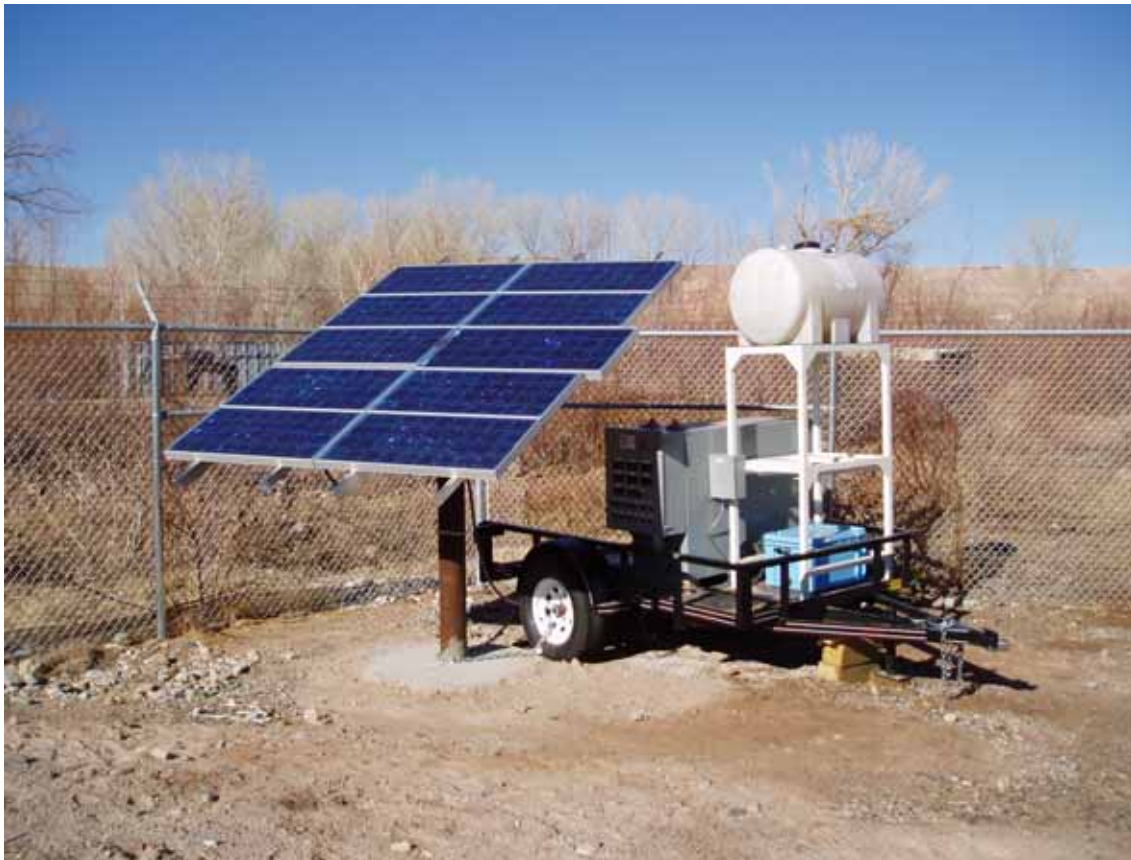
Figure 5. Setup of PVRO system in Mesquite, Nevada.
