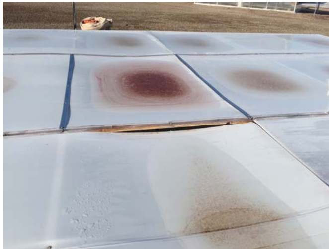
10/6/2017 PBR panel damaged by wind. Shanka fixed it with additional screws.
