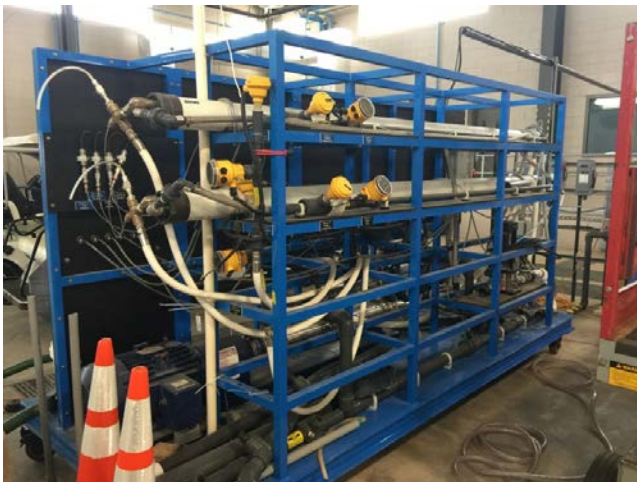
Figure 5.—RO Skid Used for the Pre-concentration of Well 1 Water.
