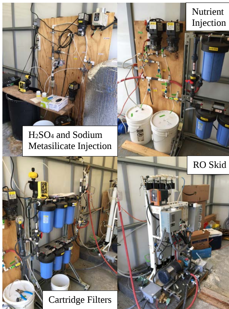
Figure 9.—Chemical injection systems, cartridge filter skid, and 2-gpm ro skid.
