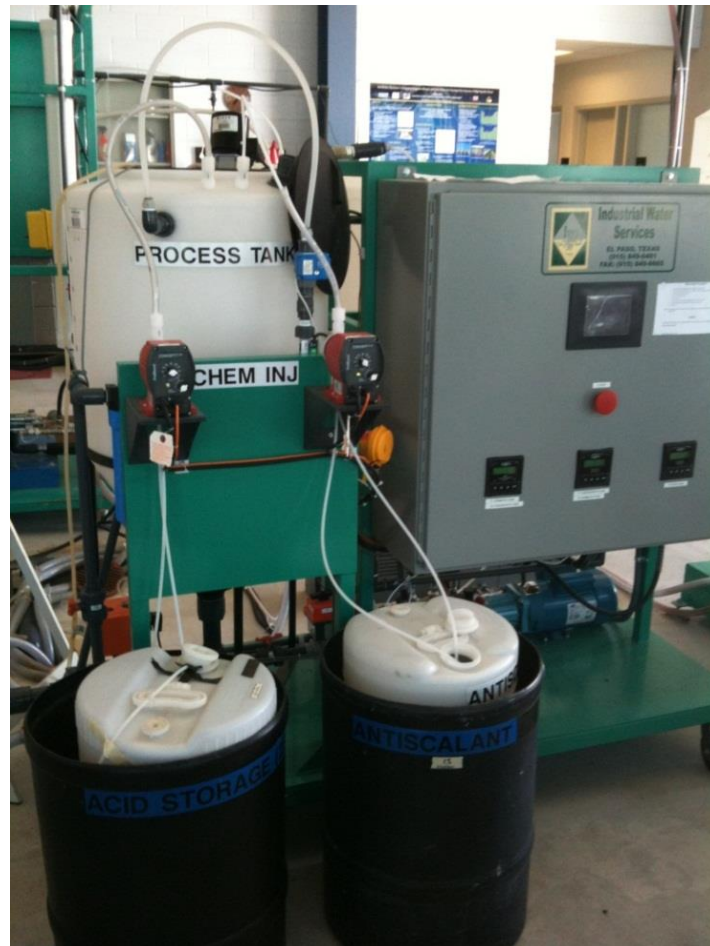
Figure 3.—Automated SWRO unit used at BGNDRF site.
