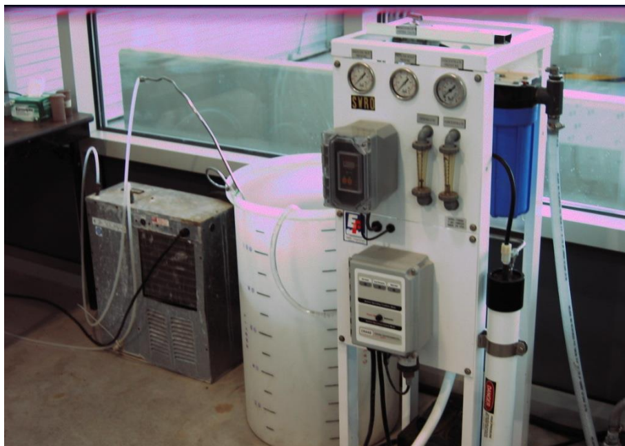
Figure 2.—SWRO unit used for conducting tests at KBH Desalting Plant.
