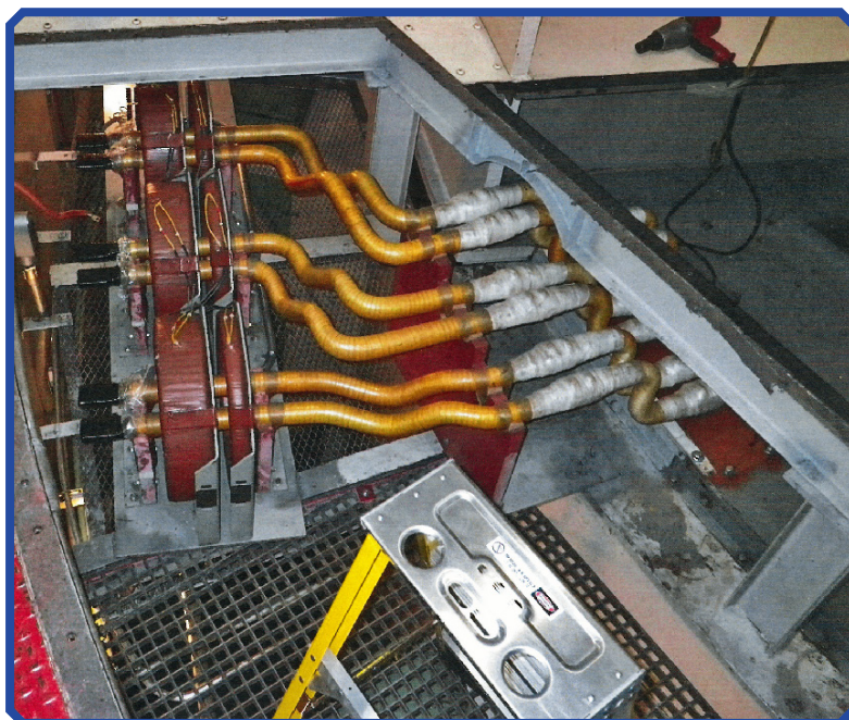
Generator neutral current transformer leads.
