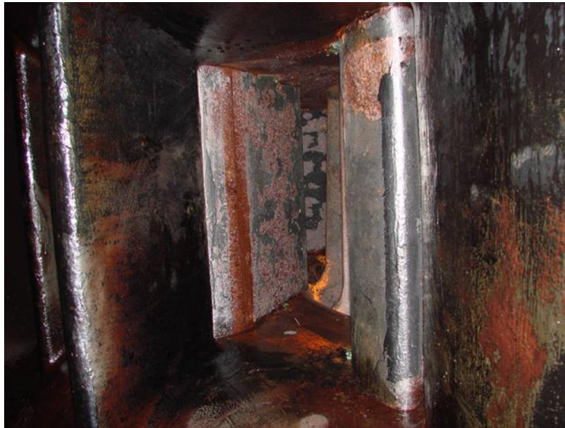
Photo 3.—Corrosion damage on wicket gates and stay vanes.
