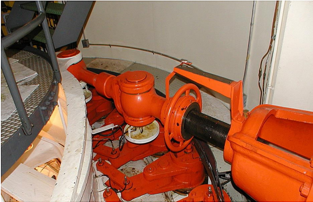
Photo 7.—Servomotor connecting rod.
