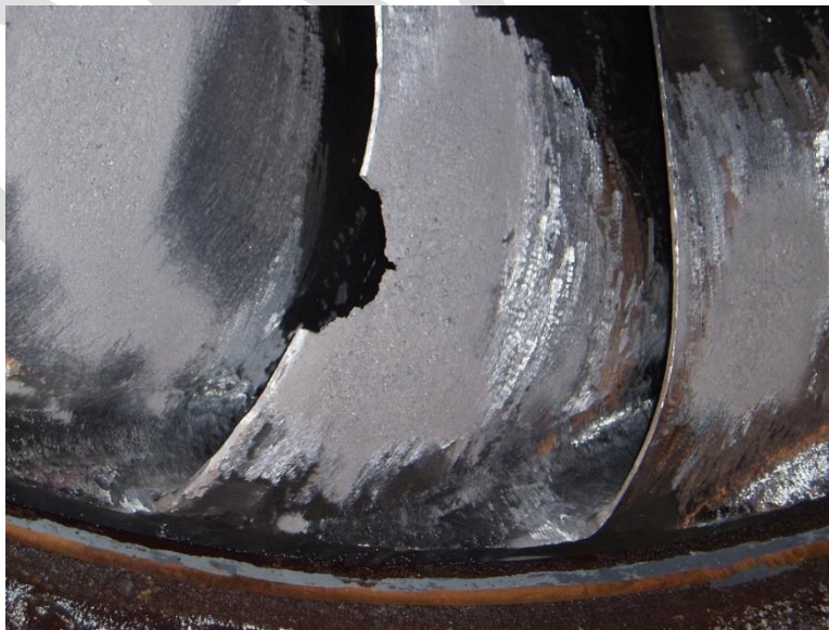
Photo 2.—Cavitation damage on turbine runner.
