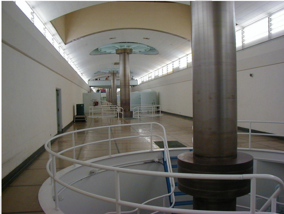
Photo 14.—Shaft and coupling.
