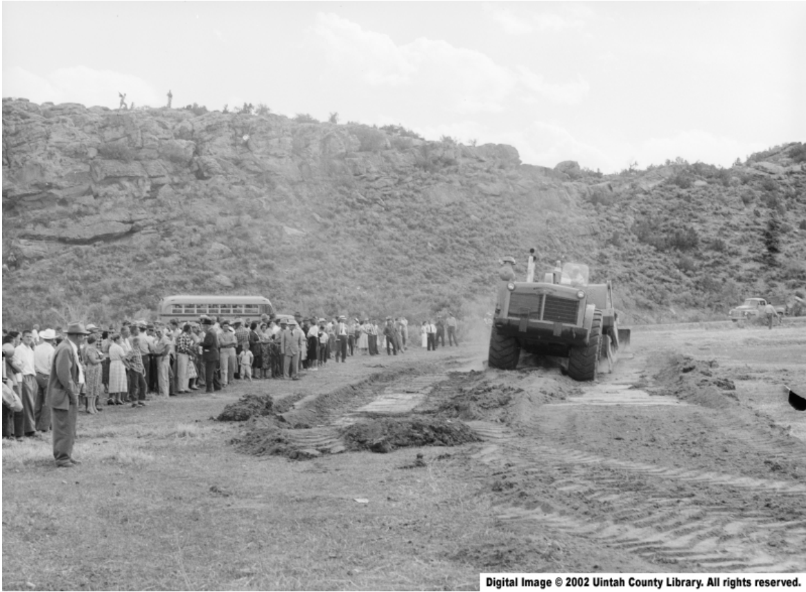
Figure 4. The guest of honor, Joseph Steinaker, for whom the dam was named, watches as a massive Euclid Scrapper turns the earth during the groundbreaking ceremony for Steinaker Dam. Mr. Steinaker had operated a farm and ranch for about sixty years at this site. Used by permission, Uintah County Regional History Center, all rights reserved.
