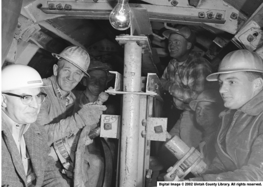
Figure 5. Crews work in the outlet tunnel arch form the first week in January, 1960. Left to right are Alton H. Peterson, Bureau of Reclamation project construction engineer; Owen Bodily, contract worker; Walter Bush contract worker; Sterling Rasmussen, contract worker; Ray Gardiner, BOR inspector; Gene Tuttle, BOR geologist. Used by permission, Uintah County Regional History Center, all rights reserved.
