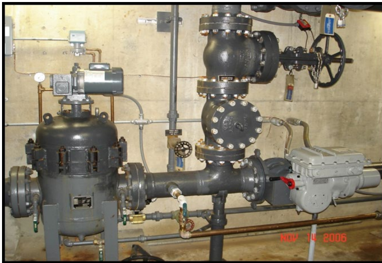
Photograph 5. Automatic, self-cleaning, moto-operated strainer and associated piping components.
