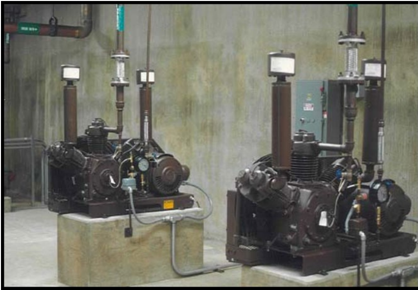
Photograph 13. Reciprocating type air compressors.
