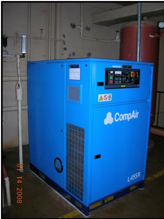
Photograph 14. Rotary screw type air compressor.
