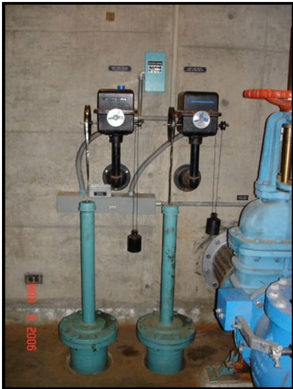
Photograph 3. Float operated sump-water-level monitoring and indicating systems.
