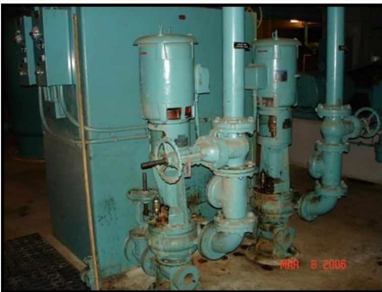
Photograph 9. Sewage pumping units and collection reservoir tank.
