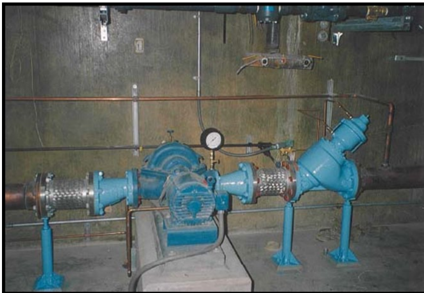
Photograph 4. Unit cooling water pump assembly.
