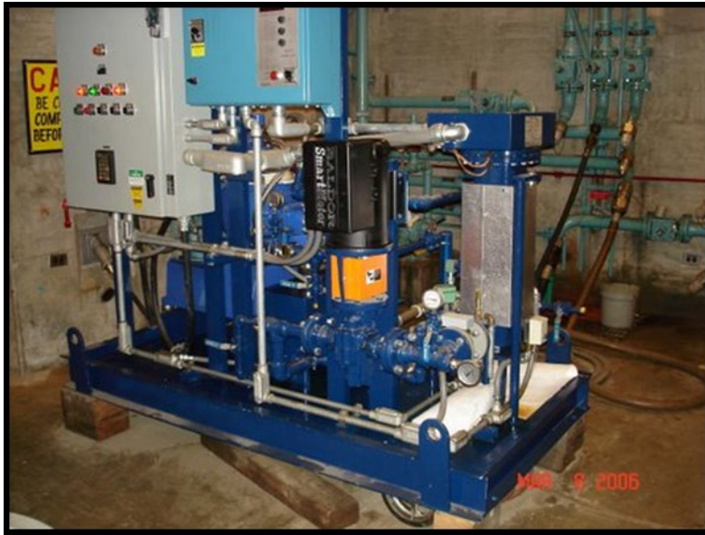
Photograph 10. Portable oil purifier equipment.
