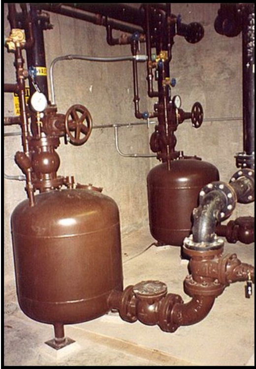
Photograph 8. Pneumatic duplex sewage ejectors.
