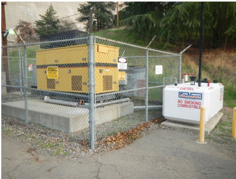
Photograph 15. Engine generator set and fuel supply tank.
