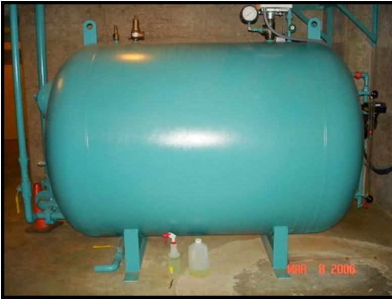
Photograph 7. Service-water hydropneumatic tank.
