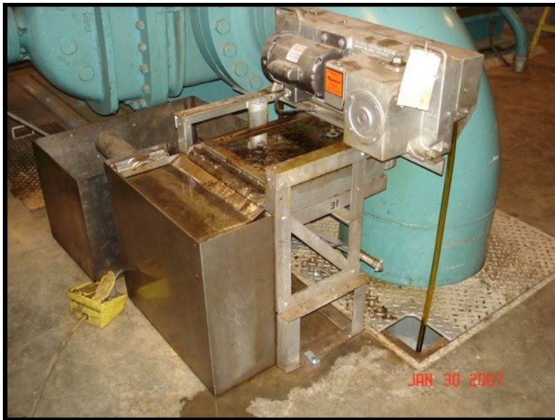
Photograph 1. Plant sump oil skimmer assembly.
