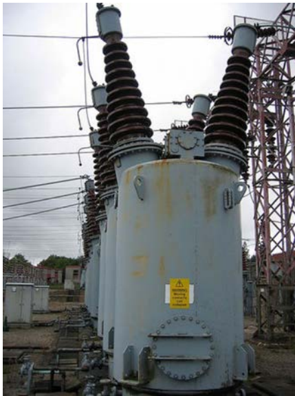
Figure 7-1. Oil circuit breaker
