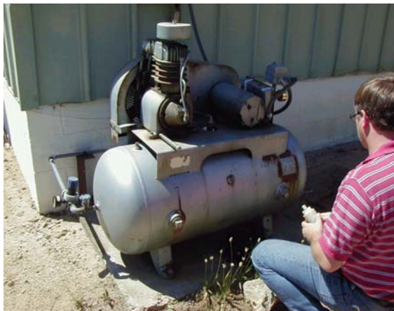
Air Receiver Tank
