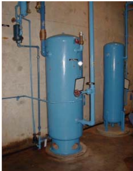
Air Receiver Tank
