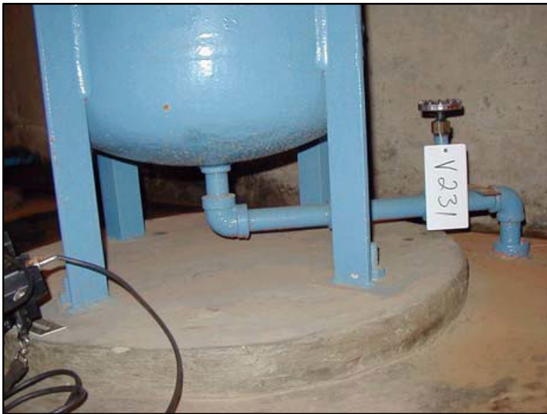
Photograph 5. Pressure vessel mounting supports.
