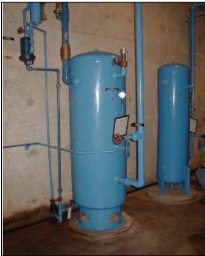
Photograph 3. Air receiver tank.
