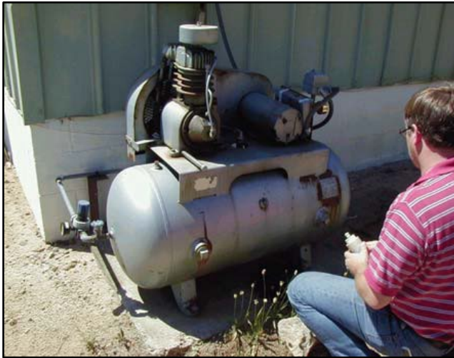
Photograph 2. Air compressor and receiver tank.
