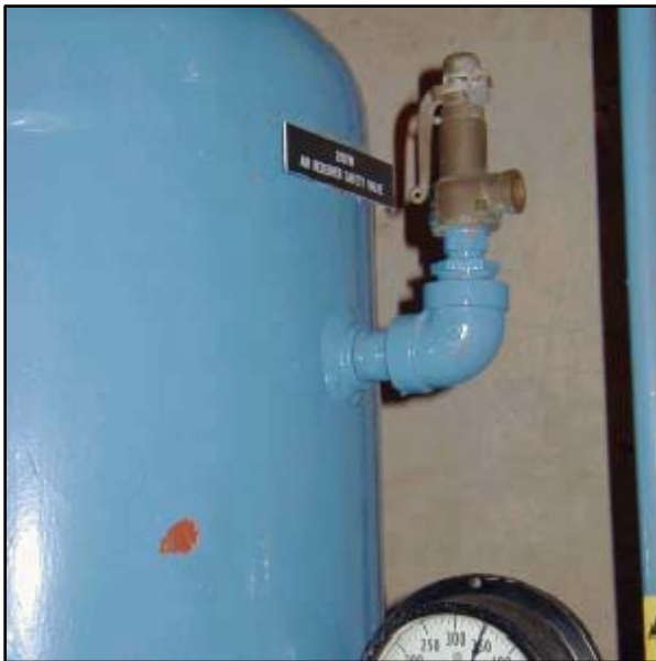
Photograph 7. Pressure relief valve.
