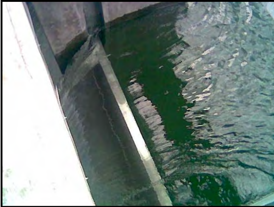
Photo 1. Flow over stoplogs
