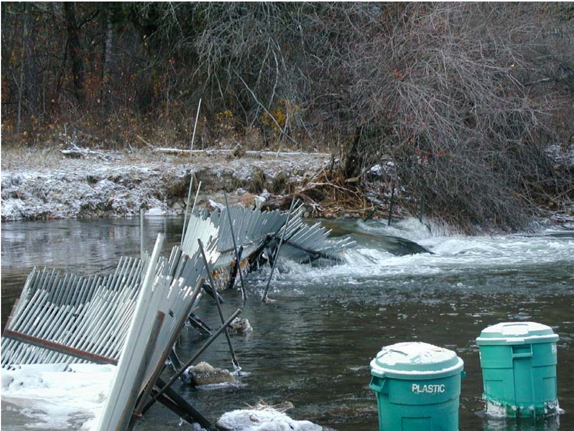
Figure 1. Middle Fork Boise River weir after snow and ice storm 11/01/03
