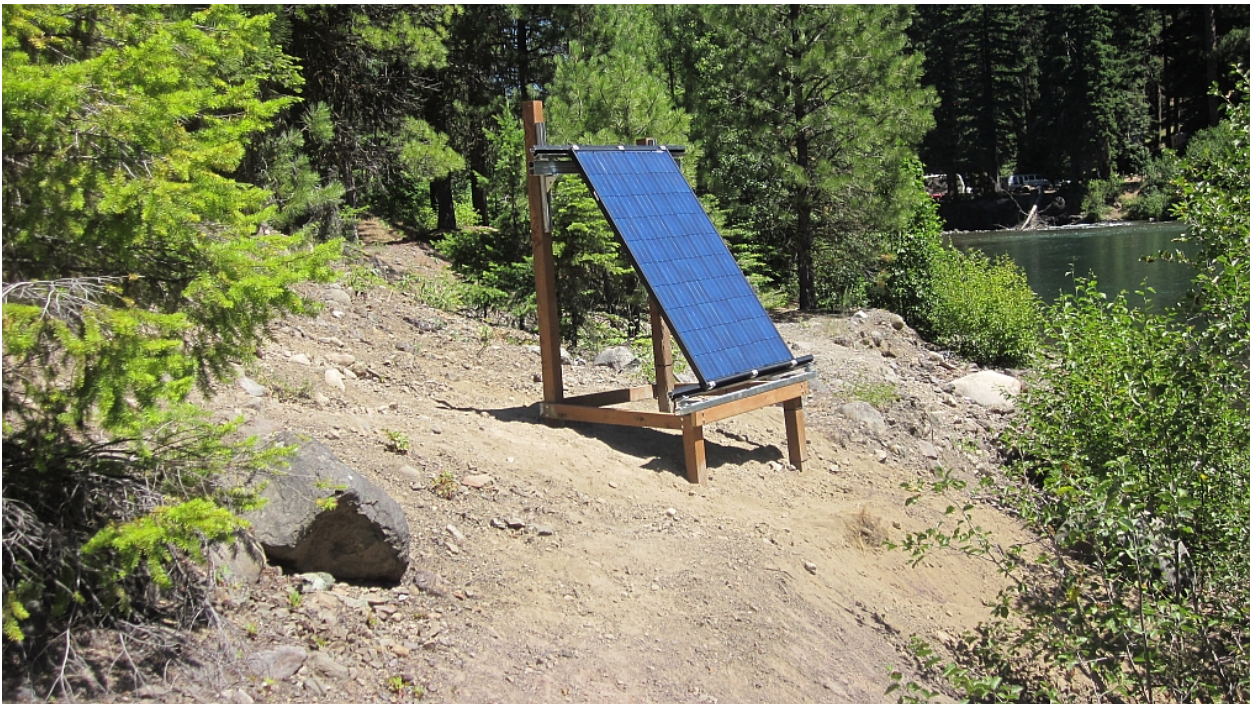
Figure 5. Solar panels installed to power the lower spillway antenna
