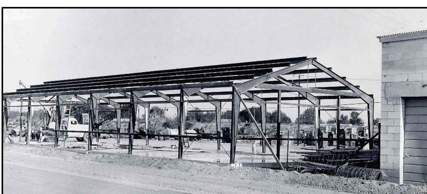
Erection of the Palisades warehouse in Rupert Yard. Photograph I-42. Courtesy A&B Irrigation District.
