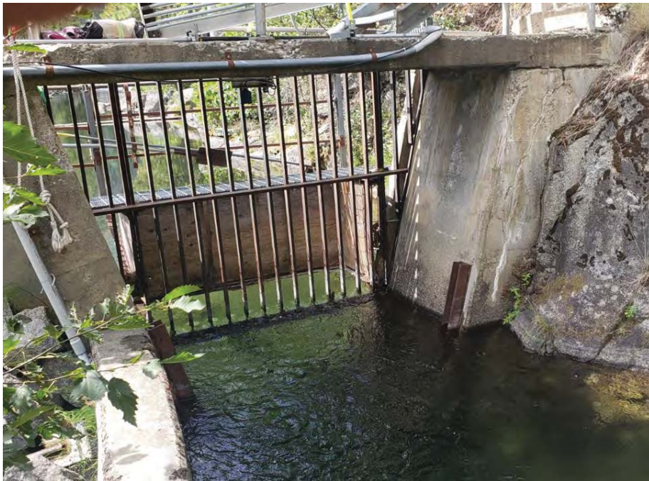
Figure 4. Looking upstream at current unscreened entrance from Icicle Creek through trash rack before entering gate house where water is diverted into a pipeline system and transported downstream to the hatchery. Photograph taken April 2019.
