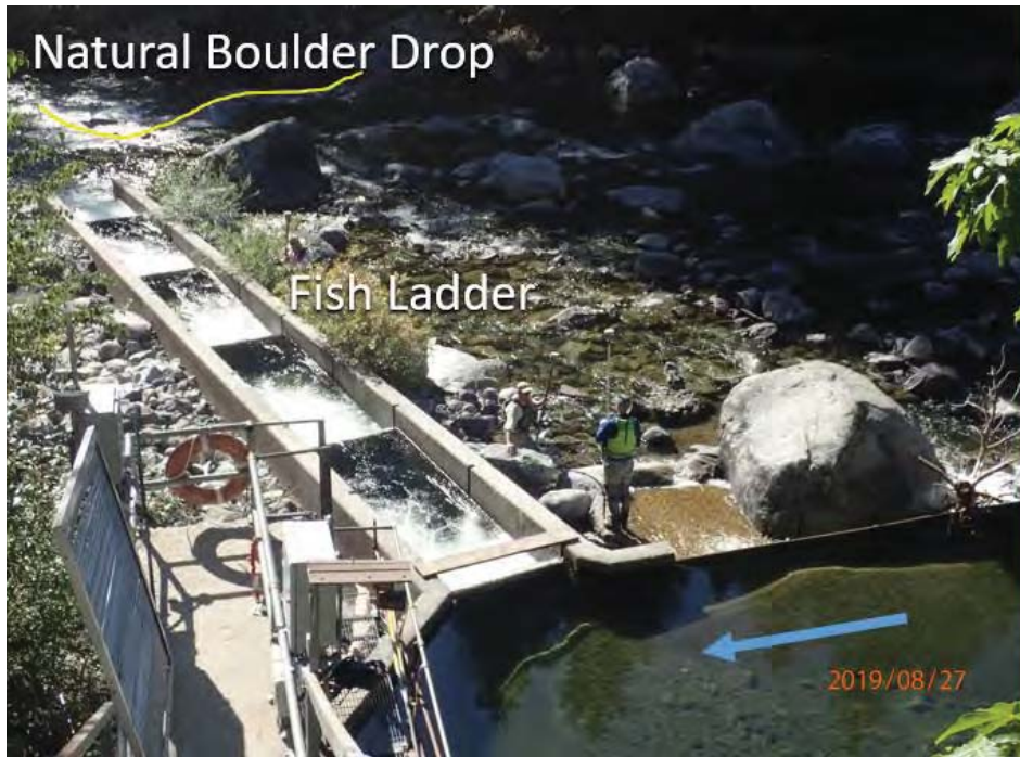
Figure 3. Existing fish ladder that was originally intended to assist with sediment sluicing. Sediment piles up in channel upstream of structure (near blue arrow) as it enters the existing intake diversion channel. The blue arrow indicates flow direction across the sluiceway. The yellow line highlights the natural boulder drop downstream. Photograph taken August 2019.
