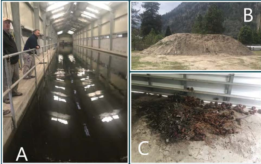
Figure 5. Sand settling basin at end of diversion pipeline (Photo A), sand removed from settling basin (Photo B), and litterfall removed from settling basin (Photo C). Photograph taken April 2019.
