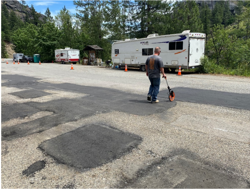
Figure 1. Existing Road Conditions on Icicle Creek Road, West of Snow Lakes Trailhead Parking Area
