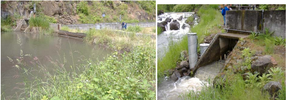
Measured sluice outlet for bypass flow at Sweetwater diversion dam. Water is flowing over compound weir on dam crest at upper left.
