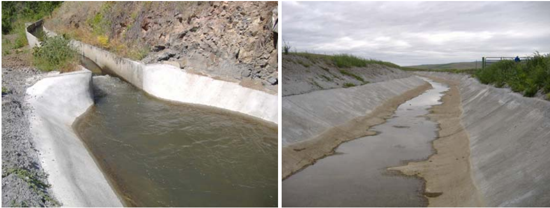
Measuring flume in transition from original bench flume to lined section of Sweetwater Canal and dewatered photo of lined Sweetwater Canal reach
