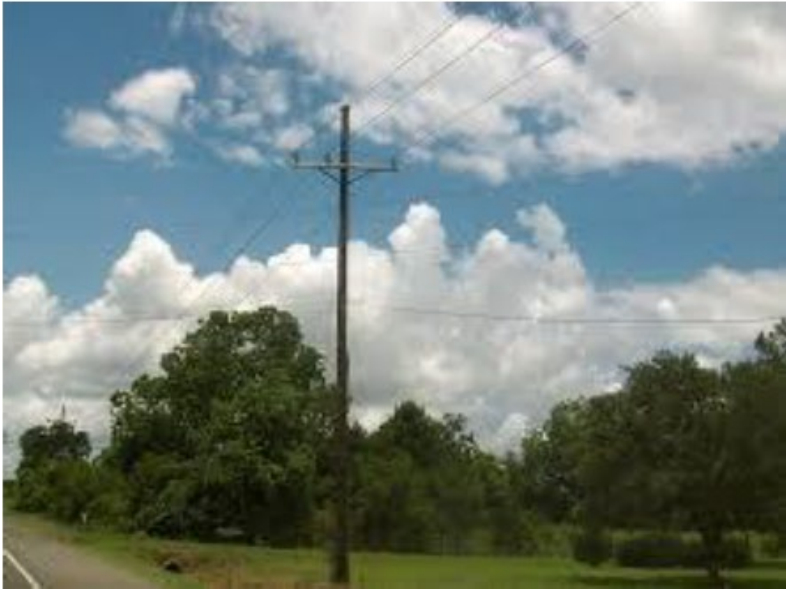
Figure A-4. Typical northern transmission line 34.5 kilovolt structure
