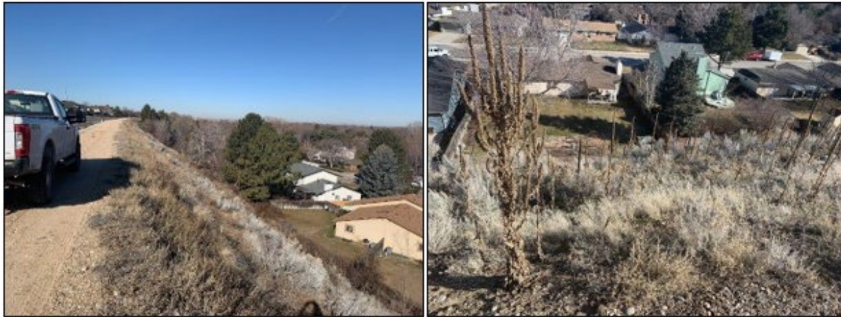
Figure 1. Photographs of residential areas within the proposed 6-mile lining/relining segment of the New York Canal. The photograph on the left illustrates a high embankment in relation to a residential area. The photograph on the right shows the top of the New York Canal embankment looking down toward a residential area.
