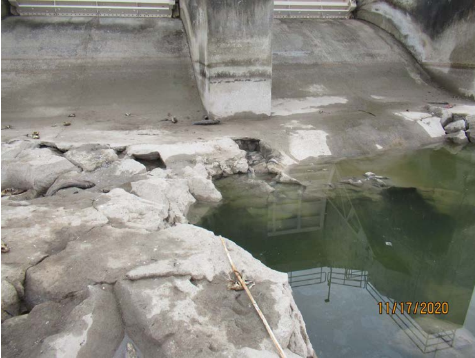
Figure 5. Erosion damage downstream of Gates 7 (left bay) and 8 (right bay)
