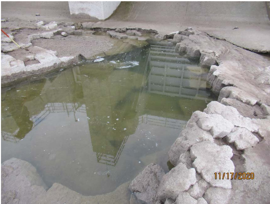
Figure 2. Erosion damage downstream of Gate 5. Damage extending into the edge of the concrete spillway apron is visible at the top of the frame.
