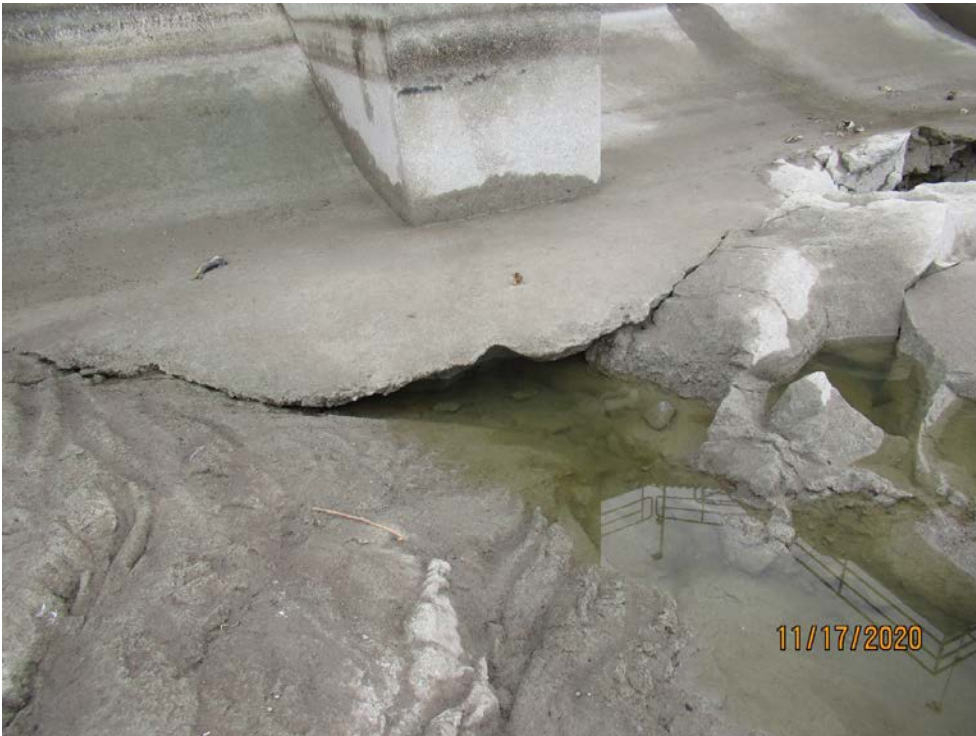
Figure 6. Erosion damage downstream of Gate 11. Undercutting of the concrete spillway apron is prominent.
