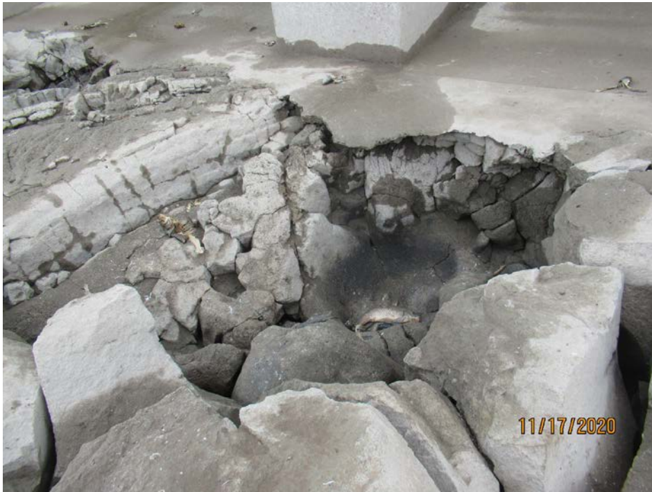
Figure 4. Erosion damage downstream of Gate 7. Damage to and undercutting of the concrete spillway apron is visible.
