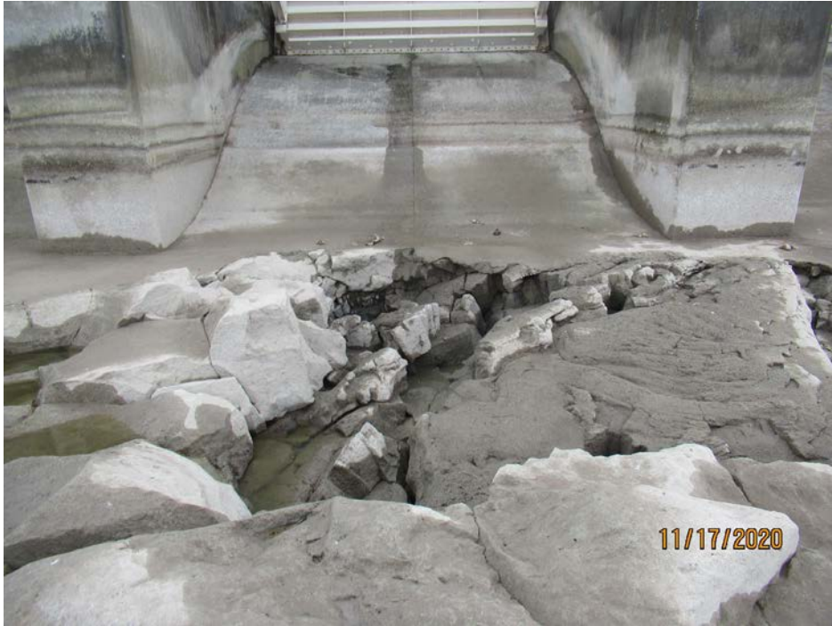
Figure 3. Erosion damage downstream of Gate 6. Damage extending into the edge of the concrete spillway apron is visible mid-photo.
