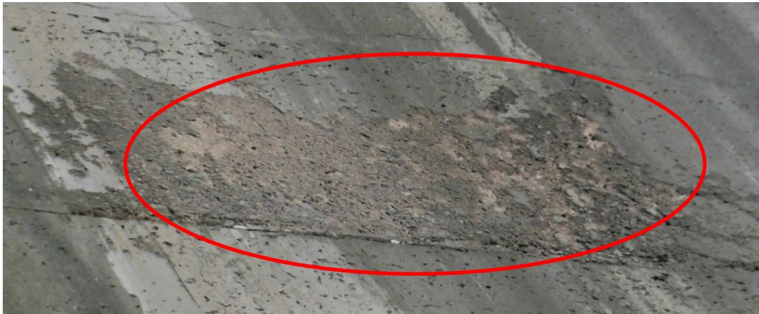
Figure 2. Disintegrating surface concrete observed on the dam face (circled).
