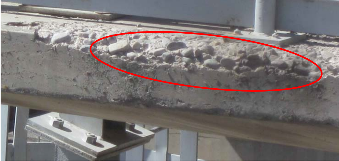
Figure 4. Structural deterioration of concrete observed on spillway gate operator deck 2. Extensive exposed aggregate is apparent (circled).
