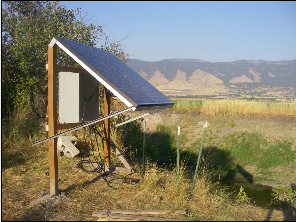
Fig. 3: NEMA box and solar panel installation on the bank above the Johnson site. The cabling at the base of the solar panel frame leads down to antennas that span the waterway.
