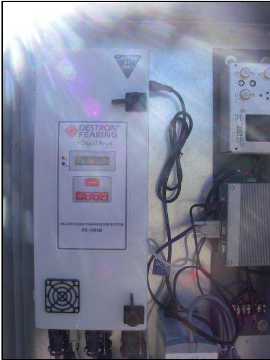
Fig. 11: Interior view of the electrical components housed within the NEMA box at Elmer Dam
