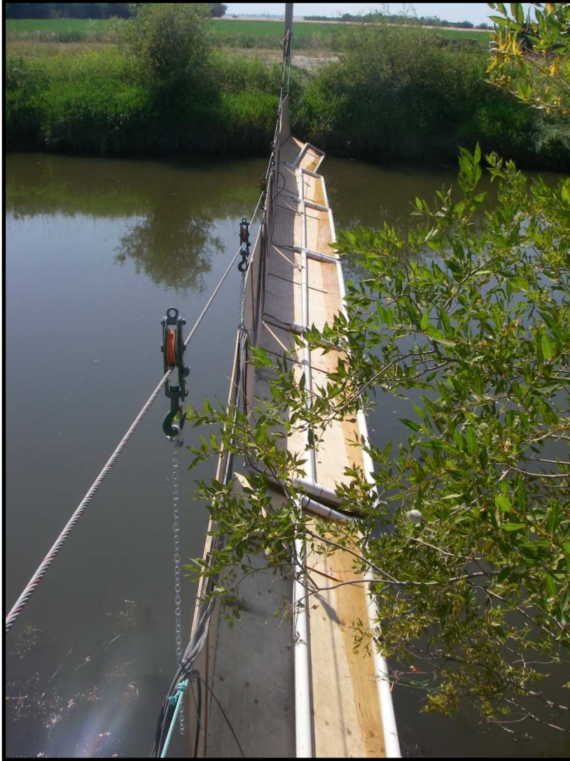
Fig. 9: Side view of the antenna configuration at Elmer Dam with antennas hanging from a steel cable crossing above the surface of the waterway.
