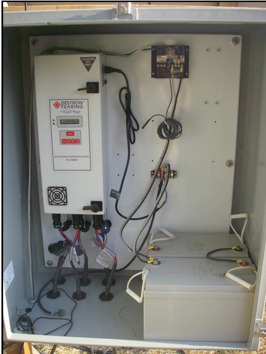
Fig. 4: Interior view of the electrical components housed within the NEMA box at the Johnson site.
