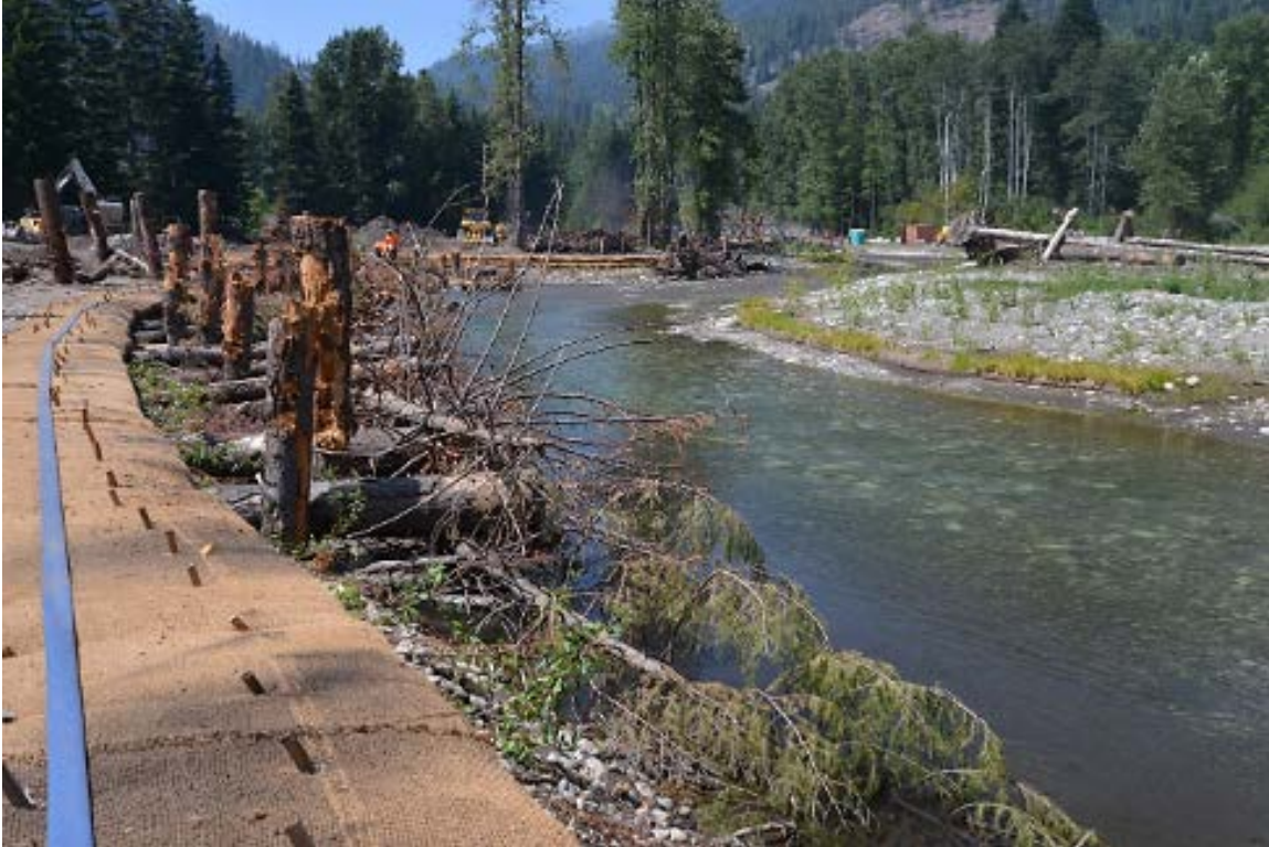
Photograph 35: Post-construction photograph shows large wood and horizontal willow plantings along the left bank of the new channel.
