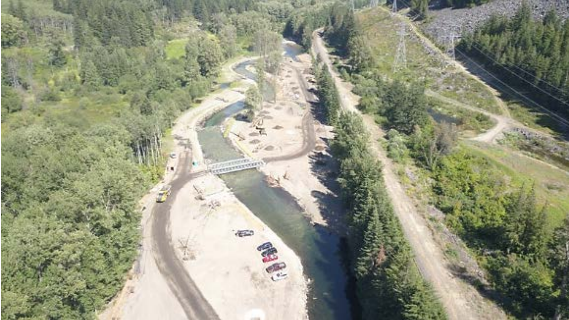
Photograph 34: Overhead view during construction after Nason Creek was diverted to the new channel.
