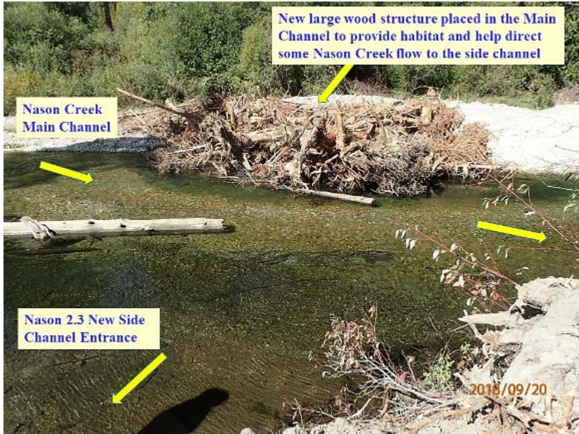
Figure 11: Post-project view shows the completed engineered log jam across Nason Creek from the side channel entrance. Flow is from left to right.
