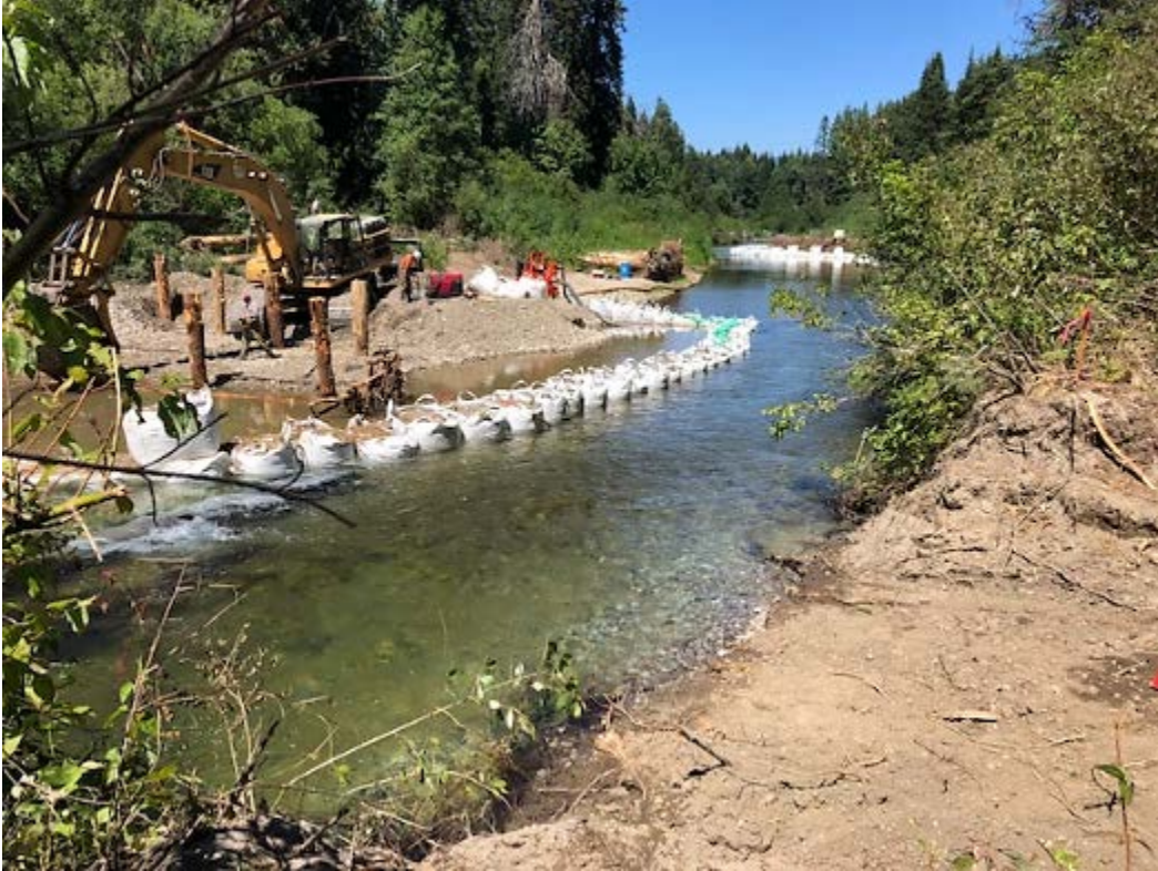
Photograph 31: Downstream view during construction at Nason Creek shows the two engineered log jams being installed, as well as the entrance location to the new side channel (see lower right of photograph) prior to activation.
