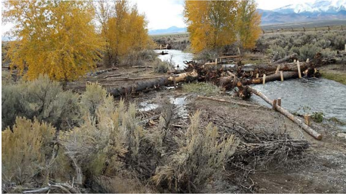
Photograph 5: Post-project view shows one of the eight channel-spanning log jams that were constructed to force water onto the floodplains at higher flows.
