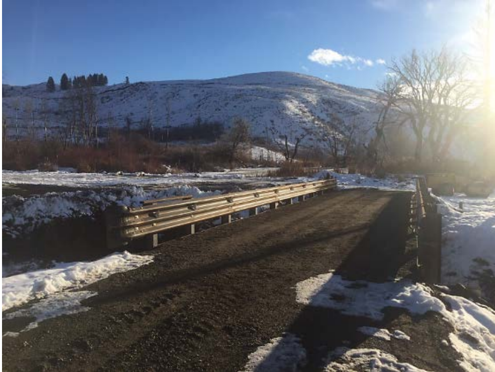
Photograph 20. Post-project view of the new channel-spanning 60 foot bridge which restores fish passage at the site
