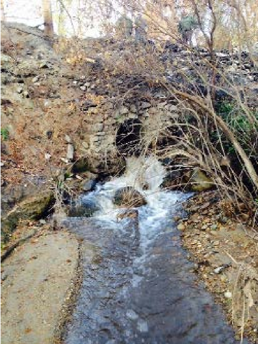
Photograph 19: Pre-project and pre-fire view of the original barrier culvert at Frazer Creek – Lazy K.
