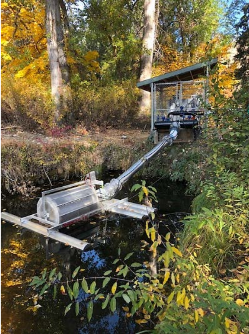
Photograph 30: Post-project view shows the newly installed fish screen on the new surface diversion from the Entiat River near the hatchery diversion.
