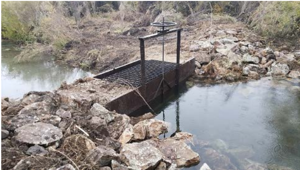
Photograph 2: Post-project view of the new Mulvaney Ditch headgate. Uncontrolled water that used to flow into the ditch is now left in Big Springs Creek. Often the additional flow into Big Springs Creek is 15 cfs.
