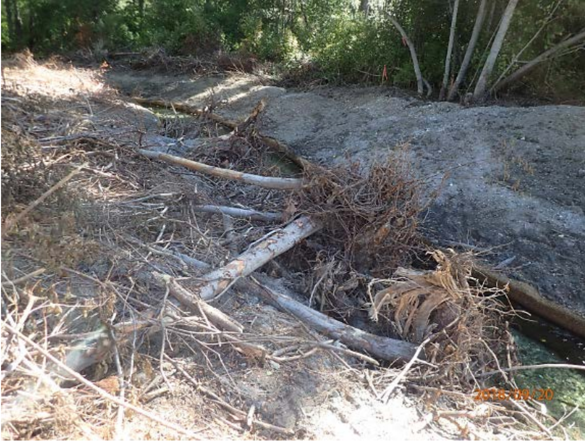
Photograph 32: Post-project view shows the completed side channel along with the newly installed large woody material. River flow is from left to right.
