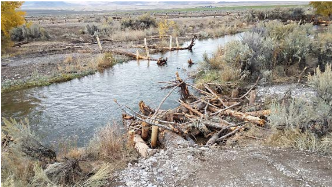
Photograph 6: Post-project view shows root wad structures that were installed to improve instream complexity and habitat. These structures ranged from single logs to seven logs. The vertical posts were driven into place to add stability to the structures.
