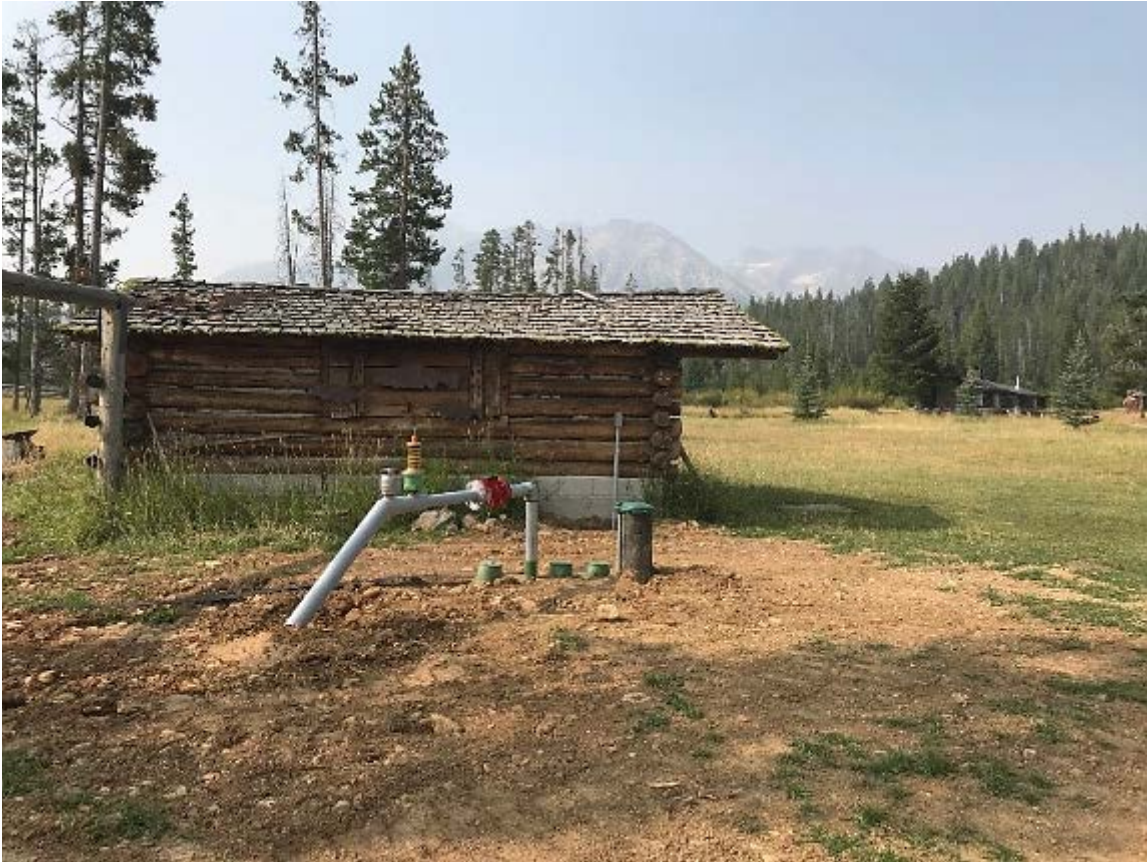
Photograph 7: Post-project view of one of the new wells drilled to provide irrigation water to small pastures. This new well allowed the elimination of the MC3 Meadow Creek diversion.
