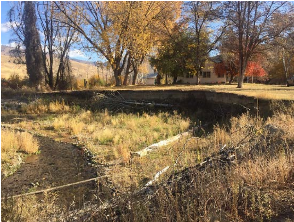
Photograph 21. Pre-project/post-fire view shows where the creek avulsed around the plugged culvert during a spring high water event.
