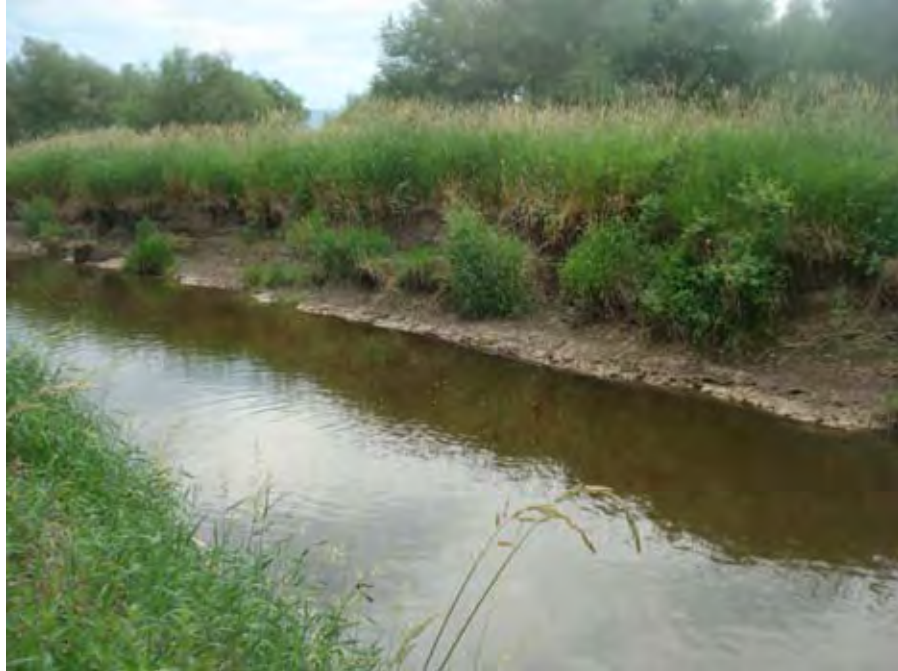
Photograph 160. View from the right bank looking upstream at slumping along the predominantly grass vegetated left bank, hard fine grained material at the toe of the bank and sand bed-load in the main channel near river mile 30.88. Reach 2 – Catherine Creek, Grande Ronde Subbasin, Oregon – Bureau of Reclamation Photograph by R. McAfee, July 28, 2010.
