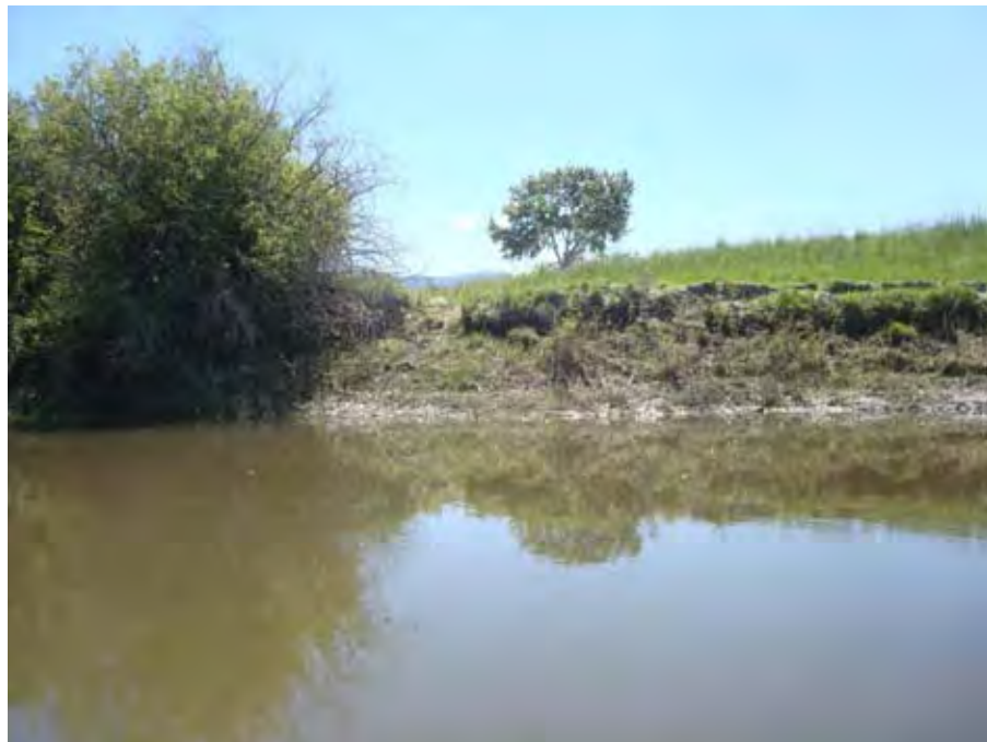
Photograph 101. View looking at grass covered levee in background, and slumping fine-grained alluvial soil (Qal2) along the left bank of Catherine Creek near river mile 1.09. Reach 1 – Catherine Creek, Grande Ronde Subbasin, Oregon – Bureau of Reclamation Photograph by D. Stelma, July 7, 2010.
