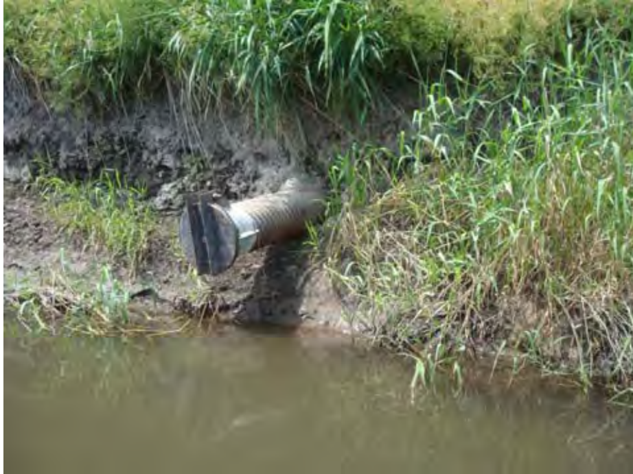
Photograph 24. View looking downstream at discharge pipe with one-way flapper valve on left bank of Catherine Creek near river mile 17.33. Reach 1 – Catherine Creek, Grande Ronde Subbasin, Oregon – Bureau of Reclamation Photograph by D. Stelma, July 10, 2010.
