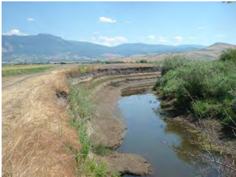
Photograph 235. View from the left bank looking downstream at the top of grass vegetated left bank and a grass/small tree vegetated right bank near river mile 26.00. Note nearly vertical denuded left bank face and the hard indurated silty sand at the toe. Reach 2 – Catherine Creek, Grande Ronde Subbasin, Oregon – Bureau of Reclamation Photograph by R. McAfee, July 29, 2010.
