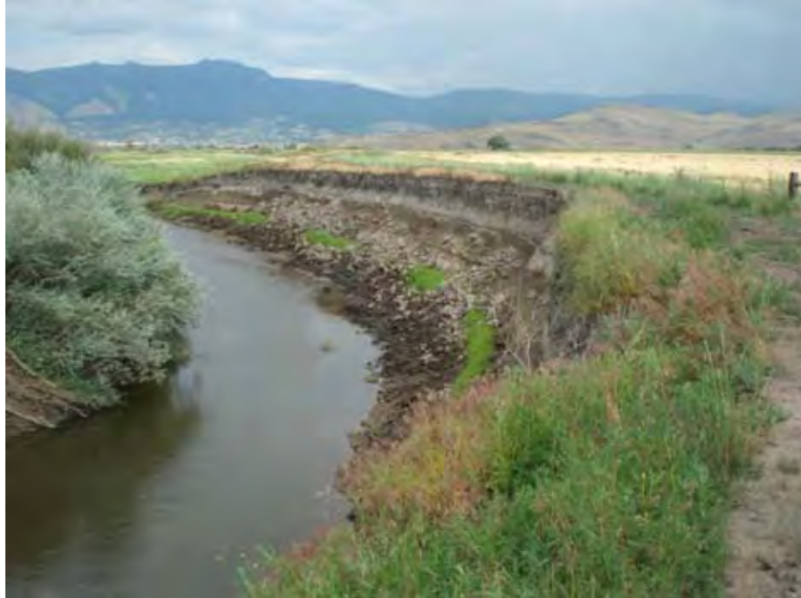
Photograph 208. View from the right bank looking downstream at a levee along the right bank that is failing near river mile 28.40. Reach 2 – Catherine Creek, Grande Ronde Subbasin, Oregon – Bureau of Reclamation Photograph by R. McAfee, July 28, 2010.
