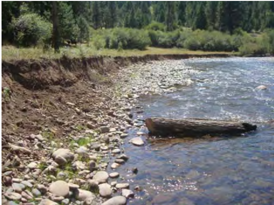
Photograph 27. View looking downstream at eroded left bank of Catherine Creek near river mile 48.31. Reach 5 – Catherine Creek, Grande Ronde Subbasin, Oregon – Bureau of Reclamation Photograph by D. Stelma, August 17, 2010.
