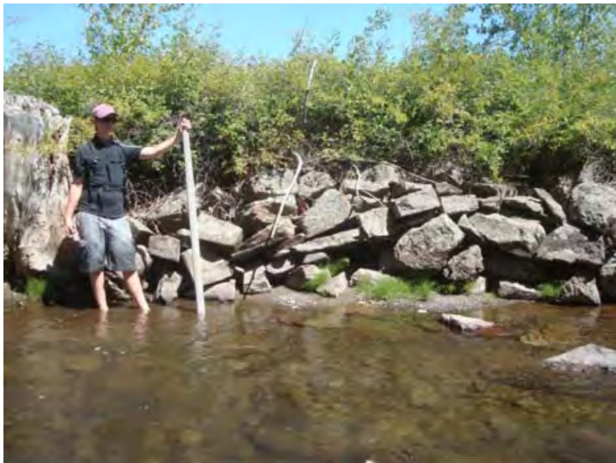
Photograph 56. View looking toward the right bank of Catherine Creek near river mile 41.26, note Oregon State (Medical Springs) Highway 203 in background, bank material consists primarily of road fill and rip rap. Reach 4 – Catherine Creek, Grande Ronde Subbasin, Oregon – Bureau of Reclamation Photograph by D. Stelma, August 16, 2010.
