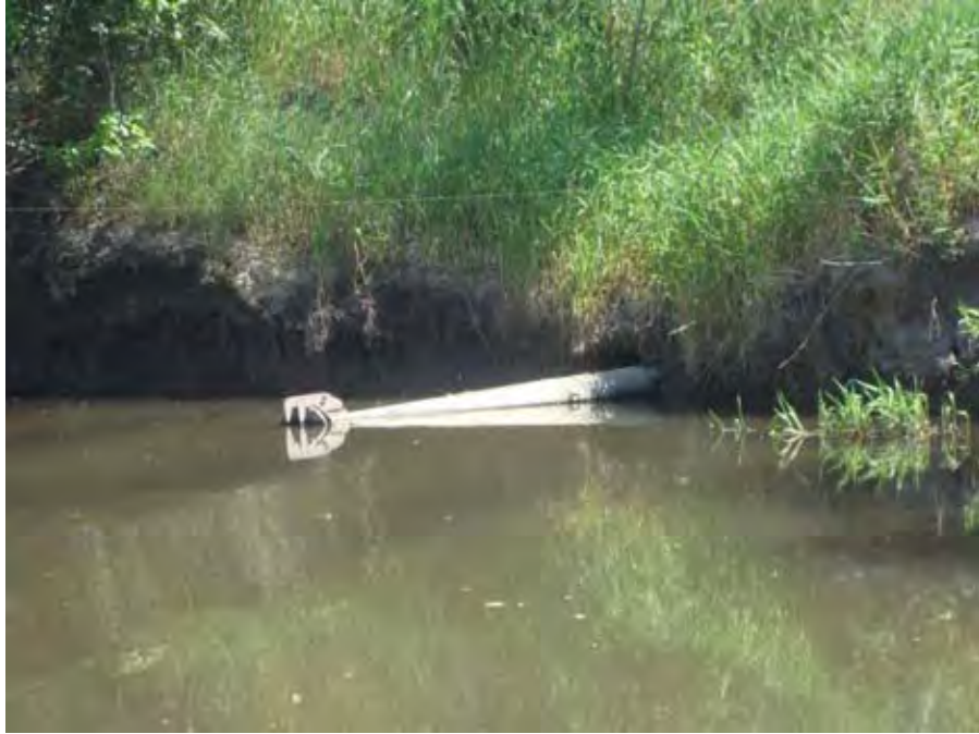
Photograph 36. Oxbow lake discharge pipe with one-way flapper valve on right (east) bank of Catherine Creek near river mile 15.55. Reach 1 – Catherine Creek, Grande Ronde Subbasin, Oregon – Bureau of Reclamation Photograph by D. Stelma, July 10, 2010.
