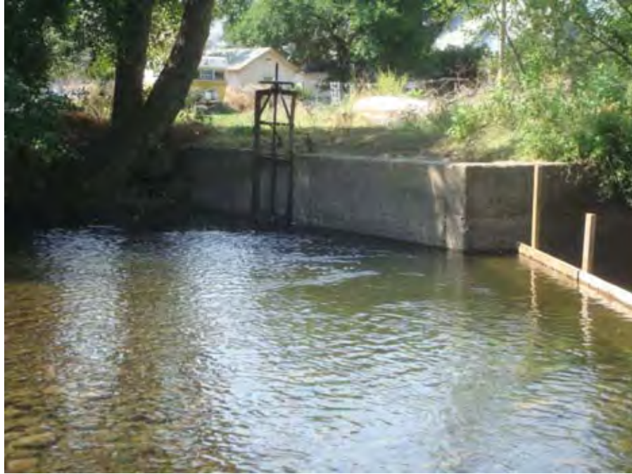
Photograph 23. View looking toward the left abutment of the diversion dam, note irrigation intake structure and slide gate, Catherine Creek channel in Union, OR near river mile 39.98. Reach 3 – Catherine Creek, Grande Ronde Subbasin, Oregon – Bureau of Reclamation Photograph by D. Stelma, August 2, 2010.
