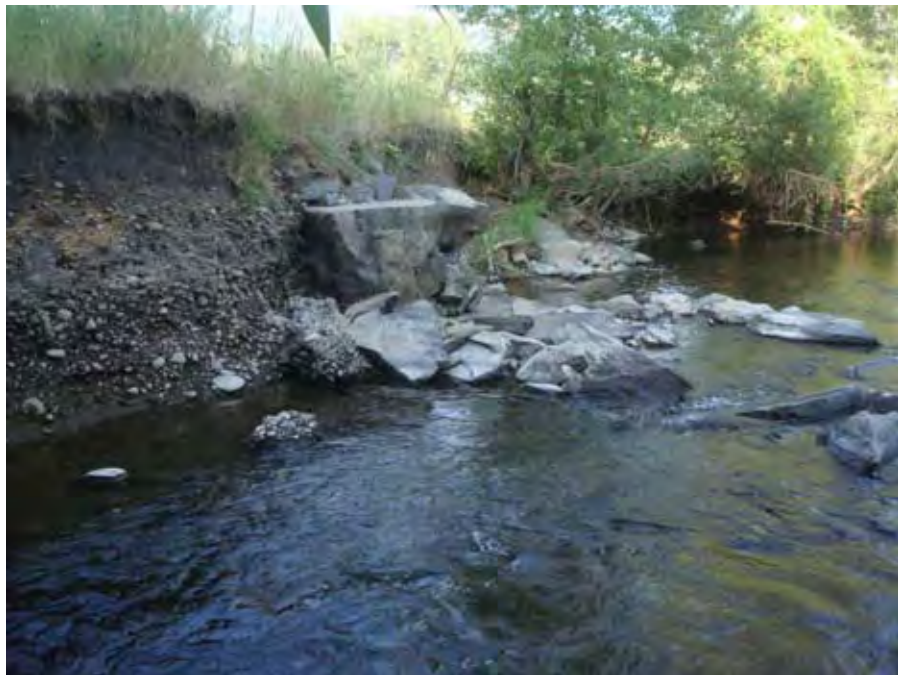
Photograph 44. View looking downstream at Catherine Creek channel near waste water treatment plant near river mile 38.90, note rip rap erosion protection along left bank. Reach 3 – Catherine Creek, Grande Ronde Subbasin, Oregon – Bureau of Reclamation Photograph by D. Stelma, August 3, 2010.
