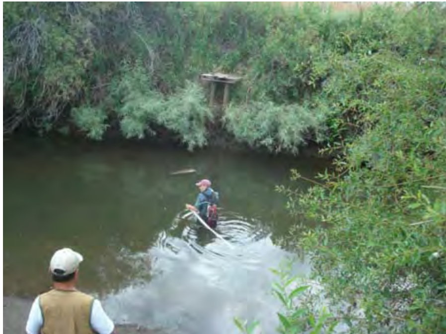
Photograph 60. View from left bank to the right showing local scour in the channel bottom and a 'diving board' along the right bank near river mile 33.89. Reach 2 – Catherine Creek, Grande Ronde Subbasin, Oregon – Bureau of Reclamation Photograph by R. McAfee, July 27, 2010.
