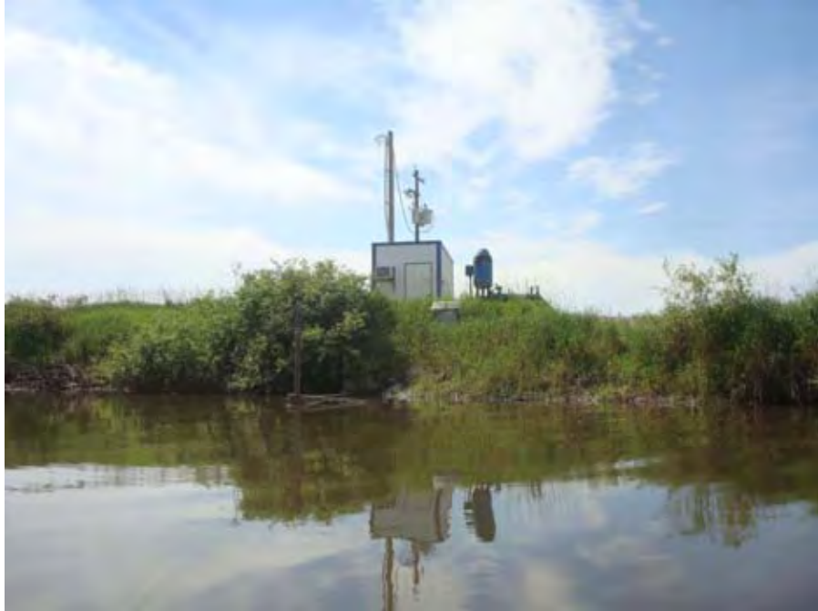
Photograph 40. Pumping plant on left (west) bank of Catherine Creek, upstream of Elmer Dam near river mile 15.13. Reach 1 – Catherine Creek, Grande Ronde Subbasin, Oregon – Bureau of Reclamation Photograph by D. Stelma, July 10, 2010.
