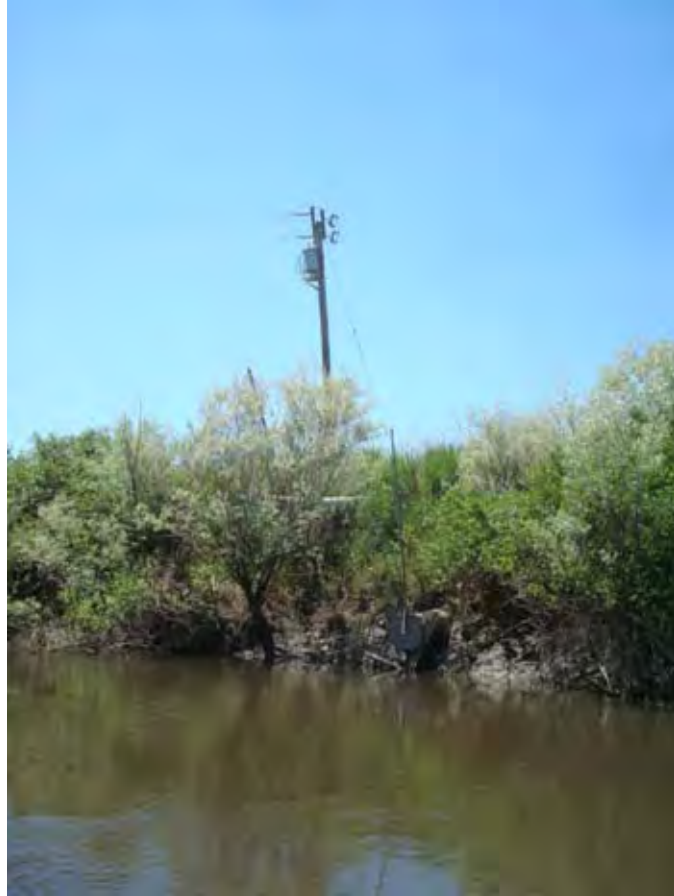
Photograph 60. View looking upstream toward the left bank at CMP drain pipe with slide-gate near river mile 12.50. Reach 1 – Catherine Creek, Grande Ronde Subbasin, Oregon – Bureau of Reclamation Photograph by D. Stelma, July 9, 2010.
