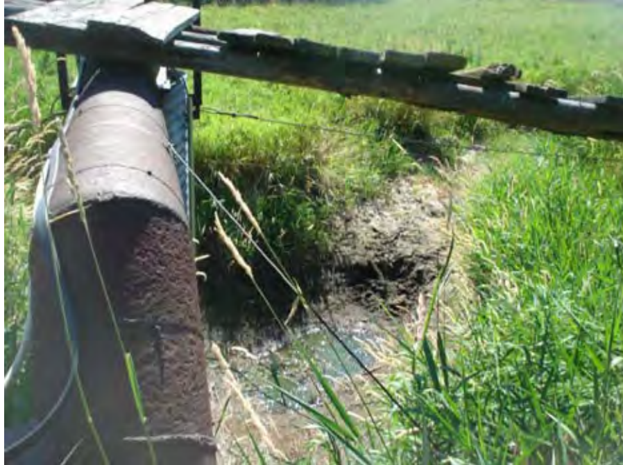
Photograph 95. View of a pump with an excavated sump on the outside of a levee set back from the right bank near river mile 32.88. Reach 2 – Catherine Creek, Grande Ronde Subbasin, Oregon – Bureau of Reclamation Photograph by R. McAfee, August 1, 2010.
