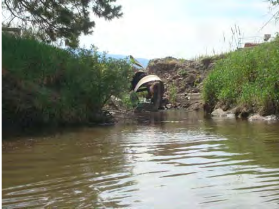
Photograph 32. Crushed culvert at discharge of man-made drainage ditch, Catherine Creek in foreground near river mile 15.77. Reach 1 – Catherine Creek, Grande Ronde Subbasin, Oregon – Bureau of Reclamation Photograph by D. Stelma, July 10, 2010.
