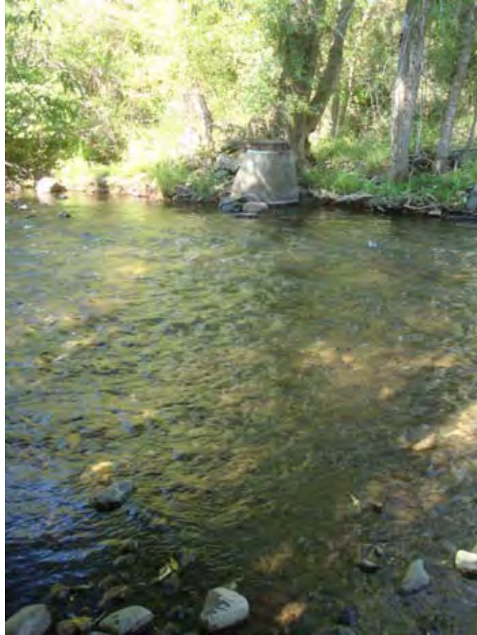
Photograph 27. View looking from left to right across Catherine Creek at manhole structure near river mile 42.57. Reach 4 – Catherine Creek, Grande Ronde Subbasin, Oregon – Bureau of Reclamation Photograph by D. Stelma, August 19, 2010.
