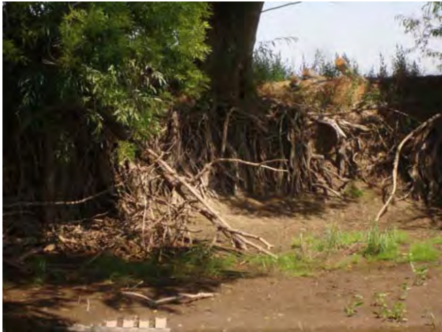
Photograph 3. View looking at under-cut and exposed tree roots on the right bank of Catherine Creek near river mile 37.14. Reach 2 – Catherine Creek, Grande Ronde Subbasin, Oregon – Bureau of Reclamation Photograph by D. Stelma, August 3, 2010.
