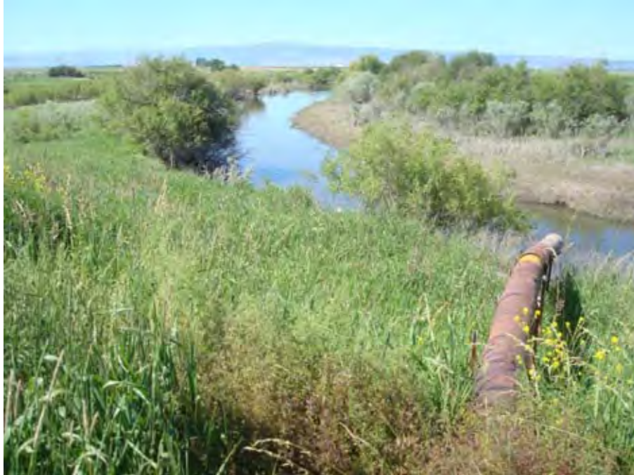
Photograph 106. View looking upstream from the crest of the levee at fabricated-barrel discharge pipe used to drain water from behind the levee, Catherine Creek in the background near river mile 0.47. Reach 1 – Catherine Creek, Grande Ronde Subbasin, Oregon – Bureau of Reclamation Photograph by D. Stelma, July 7, 2010.
