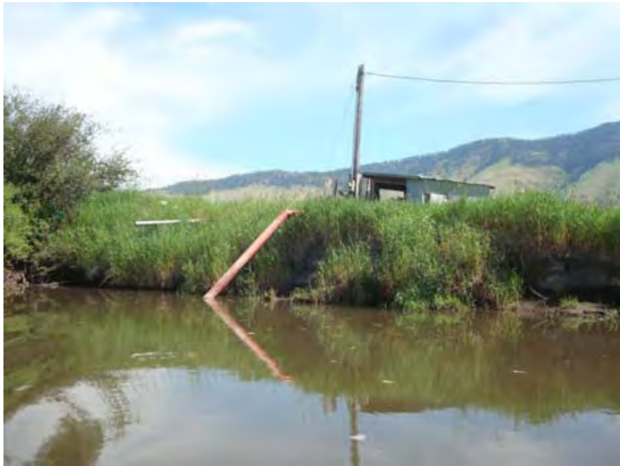
Photograph 44. View of steel pump intake pipe, Elmer Reservoir, on right bank of Catherine Creek near river mile 14.30. Reach 1 – Catherine Creek, Grande Ronde Subbasin, Oregon – Bureau of Reclamation Photograph by D. Stelma, July 10, 2010.
