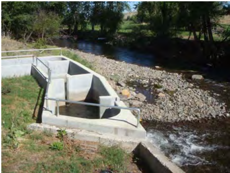
Photograph 58. Fish ladder near river mile 41.19. Reach 4 – Catherine Creek, Grande Ronde Subbasin, Oregon – Bureau of Reclamation Photograph by D. Stelma, August 16, 2010.
