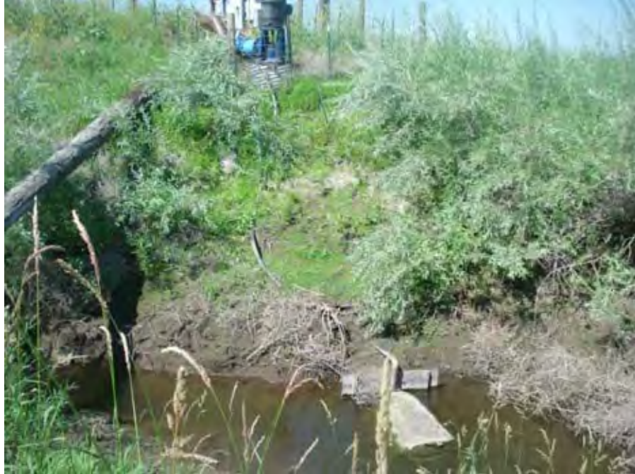
Photograph 226. View of a pump along the top of the right bank with the intake situated off the main channel, in the return channel noted in photograph 236 near river mile 27.30. Reach 2 – Catherine Creek, Grande Ronde Subbasin, Oregon- Bureau of Reclamation Photograph by R. McAfee, July 29, 2010.
