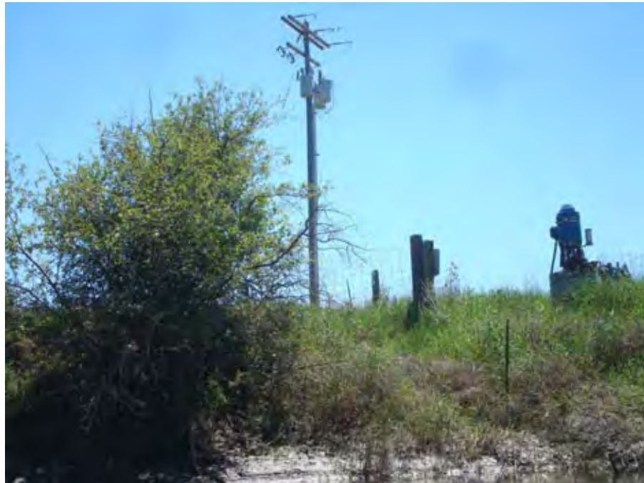
Photograph 82. View looking upstream and west at pumping plant on the east bank of Catherine Creek, intake is submerged in creek bed near river mile 7.20. Reach 1 – Catherine Creek, Grande Ronde Subbasin, Oregon – Bureau of Reclamation Photograph by D. Stelma, July 7, 2010.
