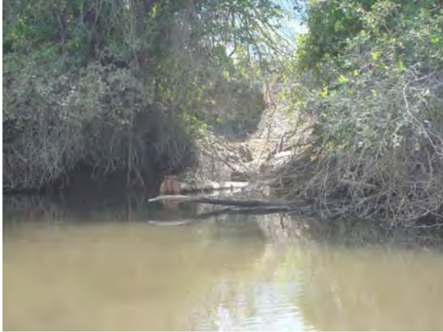
Photograph 34. Oxbow lake discharge pipe with one-way flapper valve on right (east) bank of Catherine Creek near river mile 15.67. Reach 1 – Catherine Creek, Grande Ronde Subbasin, Oregon – Bureau of Reclamation Photograph by D. Stelma, July 10, 2010.
