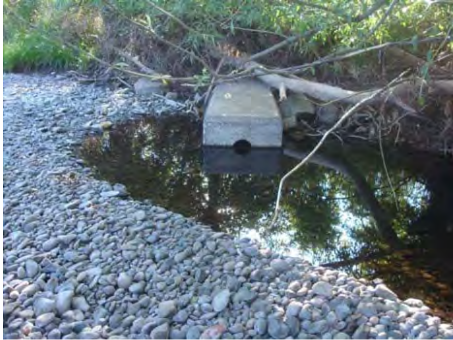
Photograph 41. View looking toward the left bank of Catherine Creek at a concrete encased discharge pipe at waste water treatment plant near river mile 39.00. Reach 3 – Catherine Creek, Grande Ronde Subbasin, Oregon – Bureau of Reclamation Photograph by D. Stelma, August 3, 2010.
