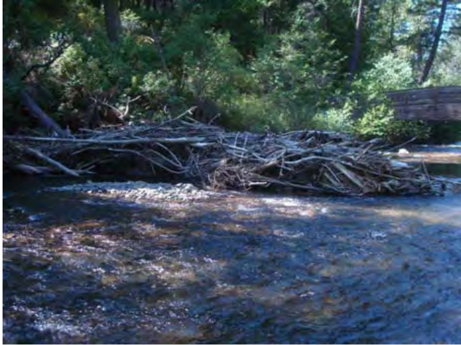
Photograph 22. View looking downstream at wood debris along the left bed and bank of Catherine Creek within Catherine Creek State Park near river mile 48.63, note left abutment of foot-bridge at upper right side of photo. Reach 5 – Catherine Creek, Grande Ronde Subbasin, Oregon – Bureau of Reclamation Photograph by D. Stelma, August 17, 2010.
