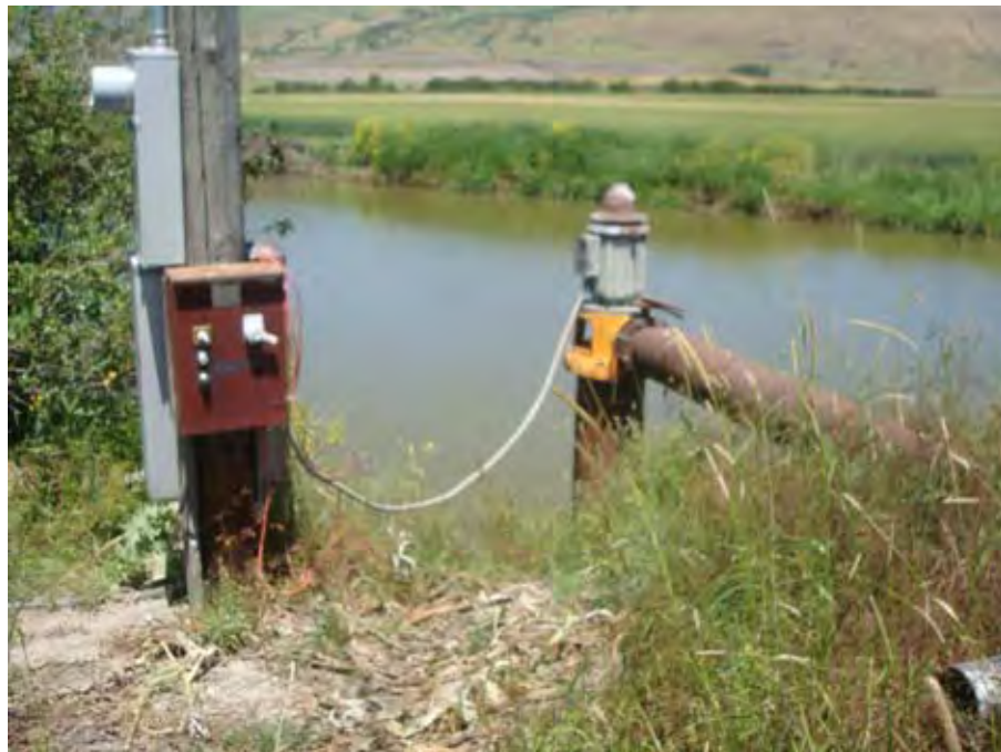
Photograph 86. Looking northeastward at cutoff meander pond and discharge pump near river mile 5.70. Reach 1 – Catherine Creek, Grande Ronde Subbasin, Oregon – Bureau of Reclamation Photograph by D. Stelma, July 7, 2010.
