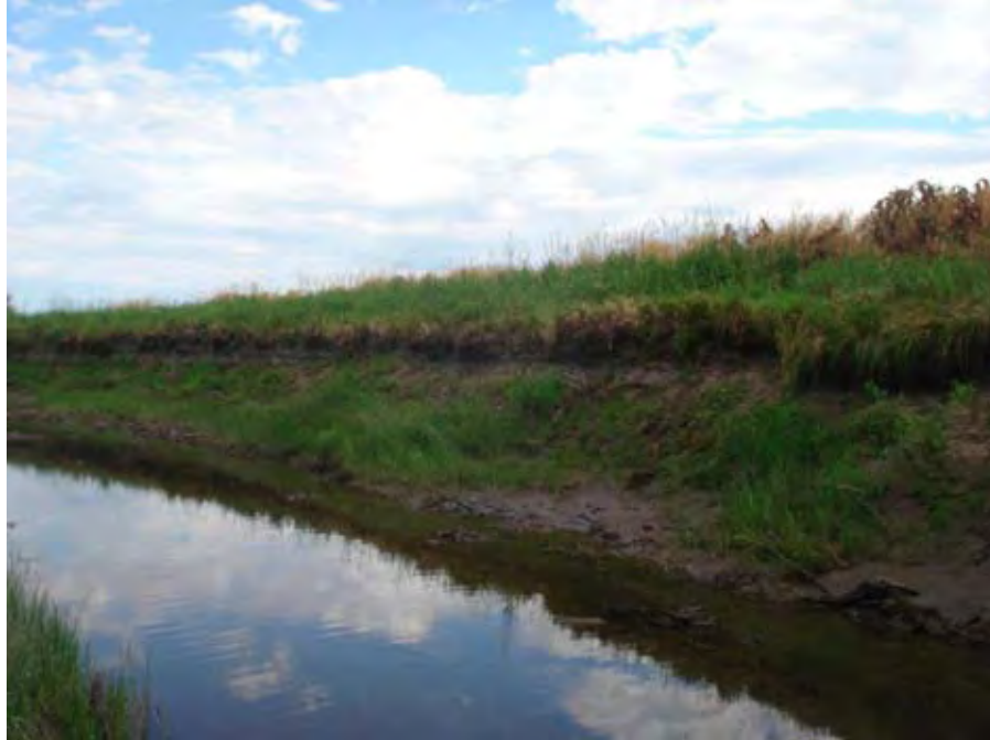
Photograph 43. View from the left bank looking downstream at grass vegetation along the top and toe of the right bank near river mile 34.33. Reach 2 – Catherine Creek, Grande Ronde Subbasin, Oregon – Bureau of Reclamation Photograph by R. McAfee, July 27 2010.
