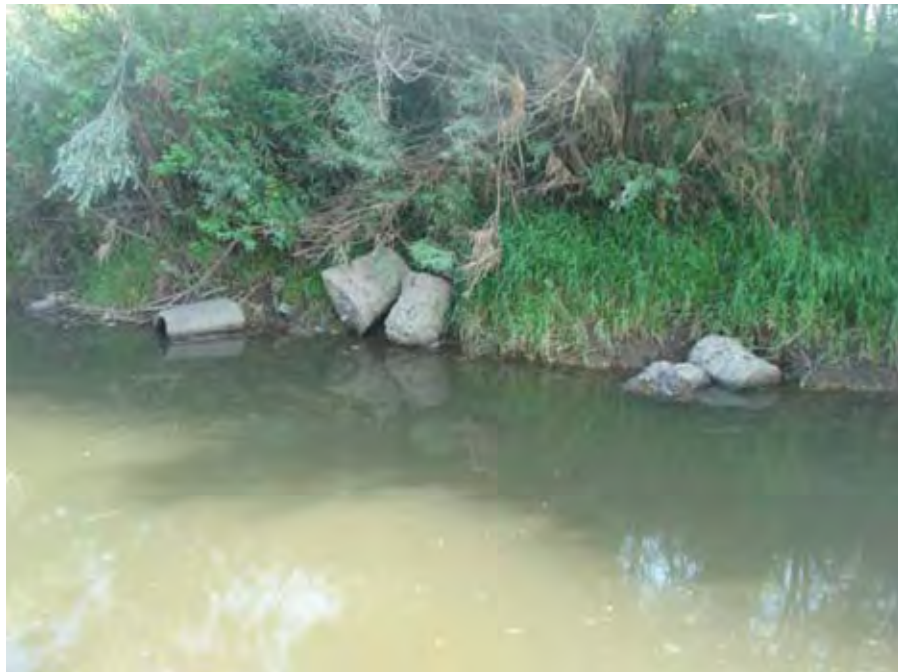
Photograph 124. View looking downstream from the left bank to the right at random concrete blocks along the toe of the right bank near river mile 31.94. Reach 2 – Catherine Creek, Grande Ronde Subbasin, Oregon – Bureau of Reclamation Photograph by R. McAfee, July 28, 2010.
