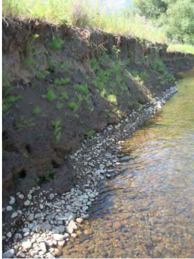
Photograph 59. View looking downstream at the left bank of Catherine Creek, note fine-grained deposits (fill or topsoil) over gravelly alluvium; this is an area where material may have been placed to artificially cut-off a stream meander in order to straighten the creek near river mile 37.77. Reach 3 – Catherine Creek, Grande Ronde Subbasin, Oregon – Bureau of Reclamation Photograph by D. Stelma, August 3, 2010.
